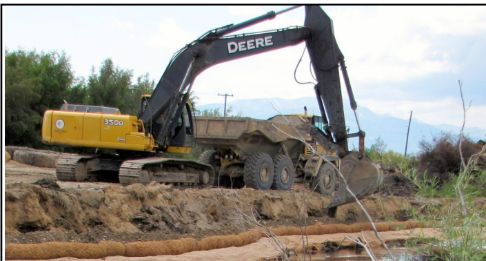
Stream bank rebuild in 2013 in Phase 1 (near Warm Springs). The coir logs just below the soil line are no longer used for bank construction, replaced by brush matrices in later phases.
