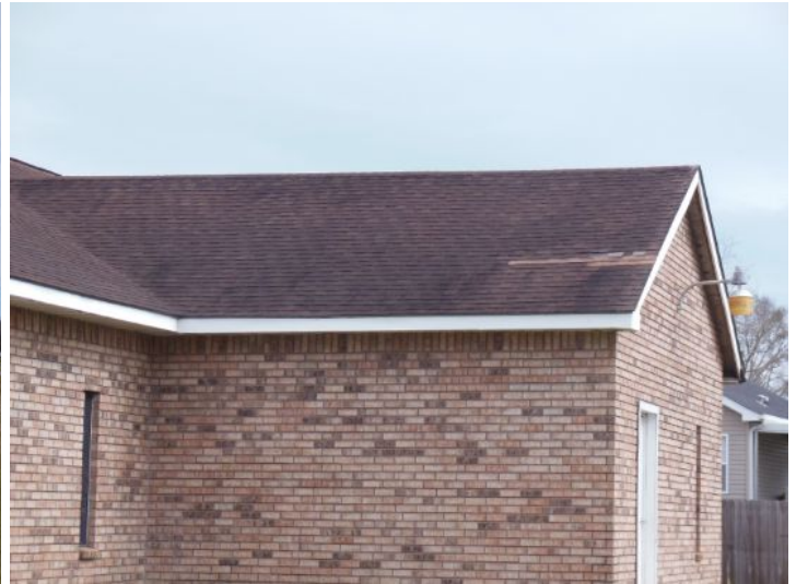
Damaged shingles at rear
