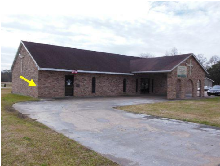
Downspout recommended here
