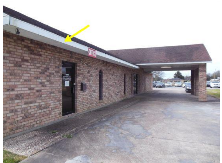
Gutters recommended here
