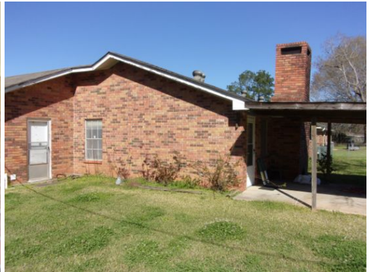
Peelings paint at fascia siding.
