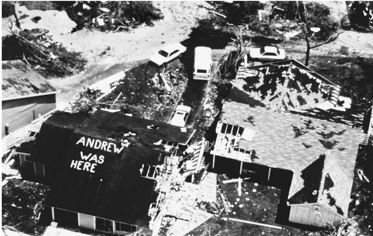
A rooftop message from a homeowner attests to the damage and destruction that can be inflicted on buildings by a tropical cyclone's prying winds and pounding rains. Hurricane Andrew swept into southern Florida in 1992 as a Category 5 hurricane. (NOAA)
