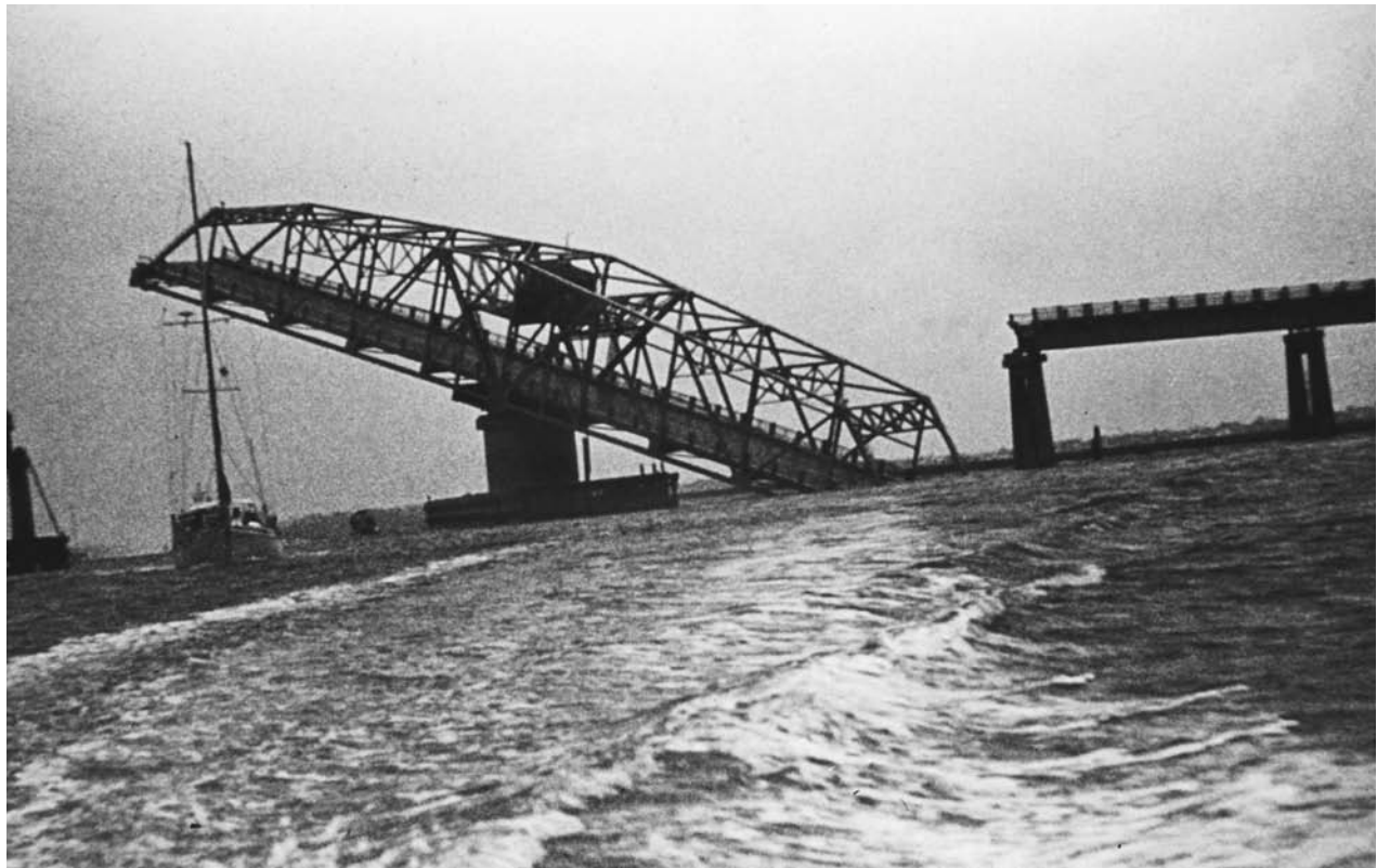
A swing bridge lies askew following Hurricane Hugo's road trip through South Carolina during the night of September 21, 1989. Photographs such as this attest to the destructive power of a tropical cyclone. (NOAA)
