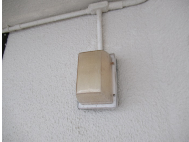
Typical exterior light fixture
