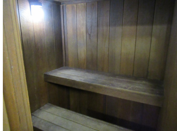
Sauna interior Note: Wood deterioration.
