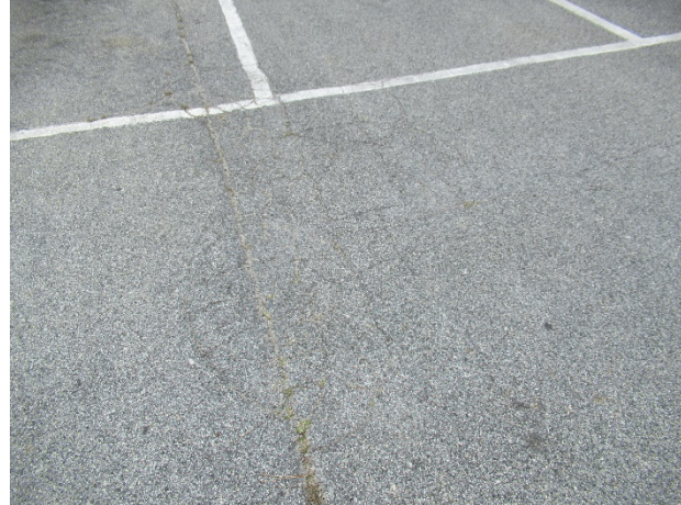
Pavement cracks and deterioration
