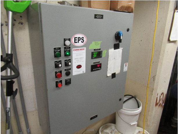
Geothermal system control panel
