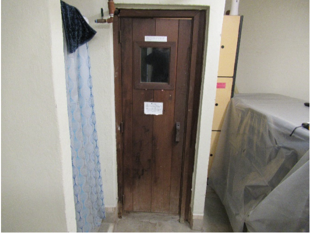
Sauna door Note: Wood deterioration.
