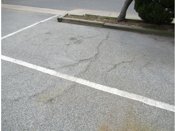
Pavement cracks and deterioration
