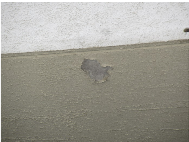
Stucco finish deterioration at soffit
