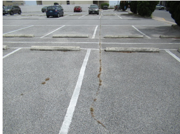
Parking area overview Note: Cracks and deterioration.
