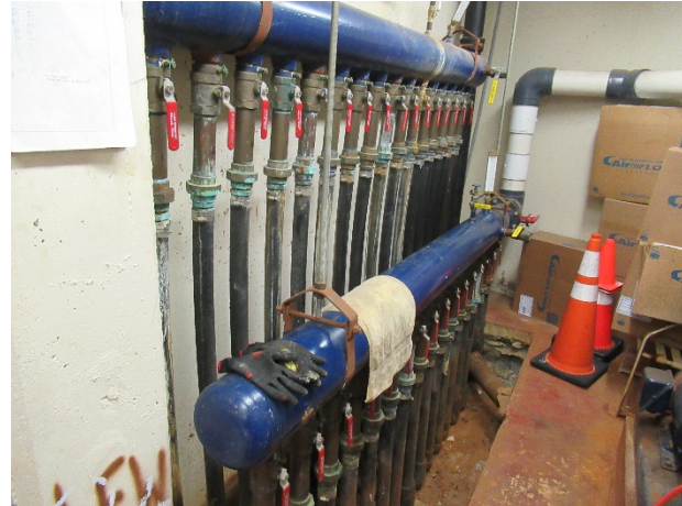
Geothermal system loop manifolds
