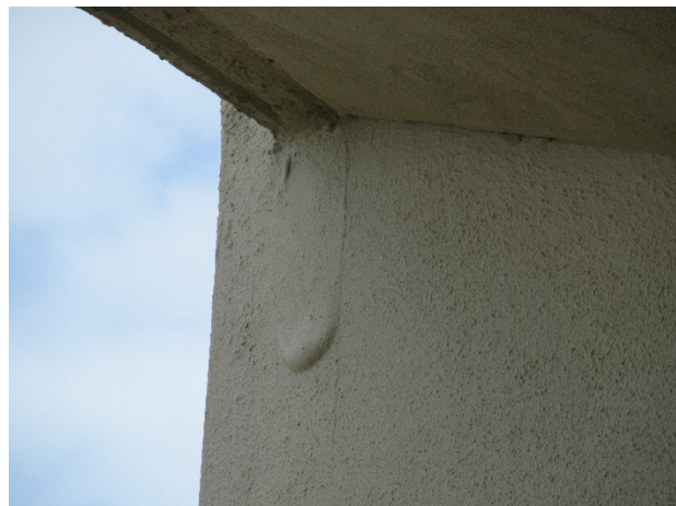
Water trapped behind stucco coating
