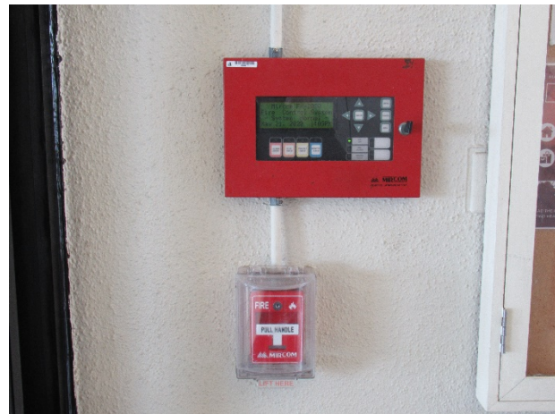
Life safety system annunciator and pull station
