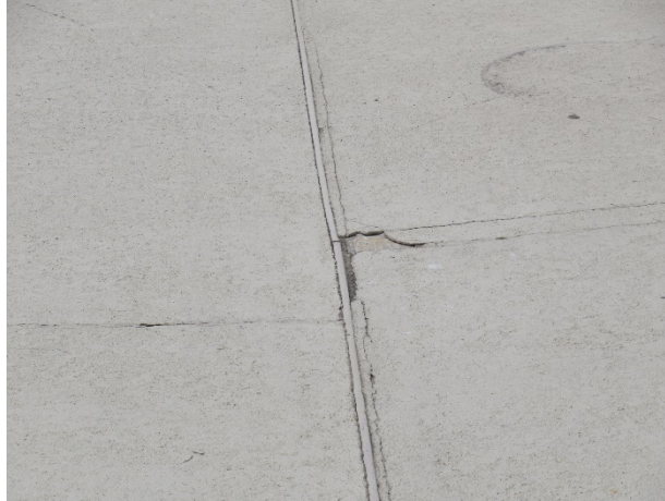
Coating deterioration and cracks
