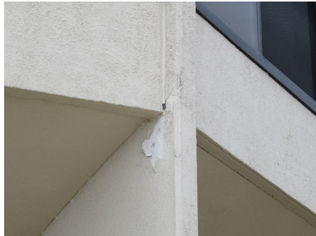
Stucco finish deterioration
