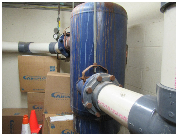
Geothermal system pressure tank
