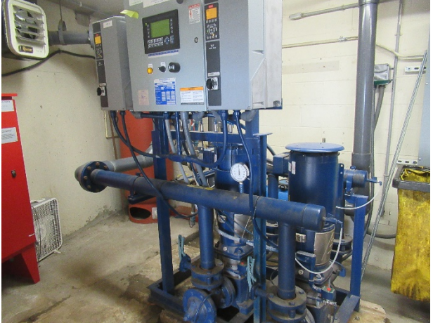
Domestic water pumps, manifold, control panel and variable frequency drives
