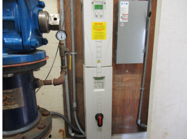
Geothermal system pump and variable frequency drives
