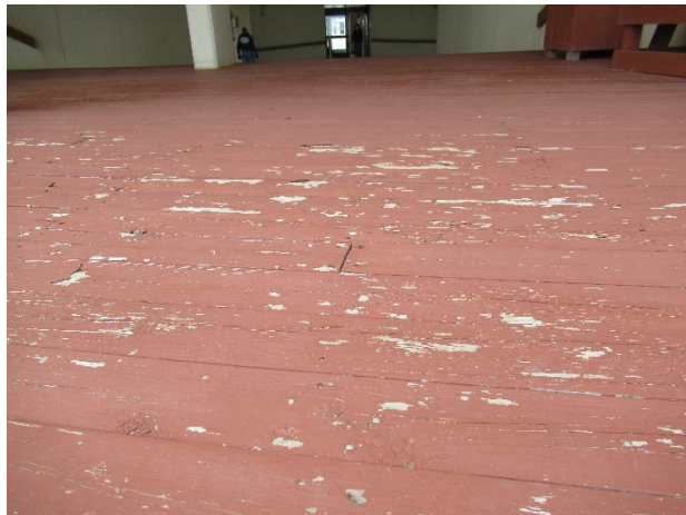
Paint finish deterioration
