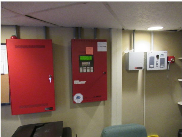
Main life safety system control panel
