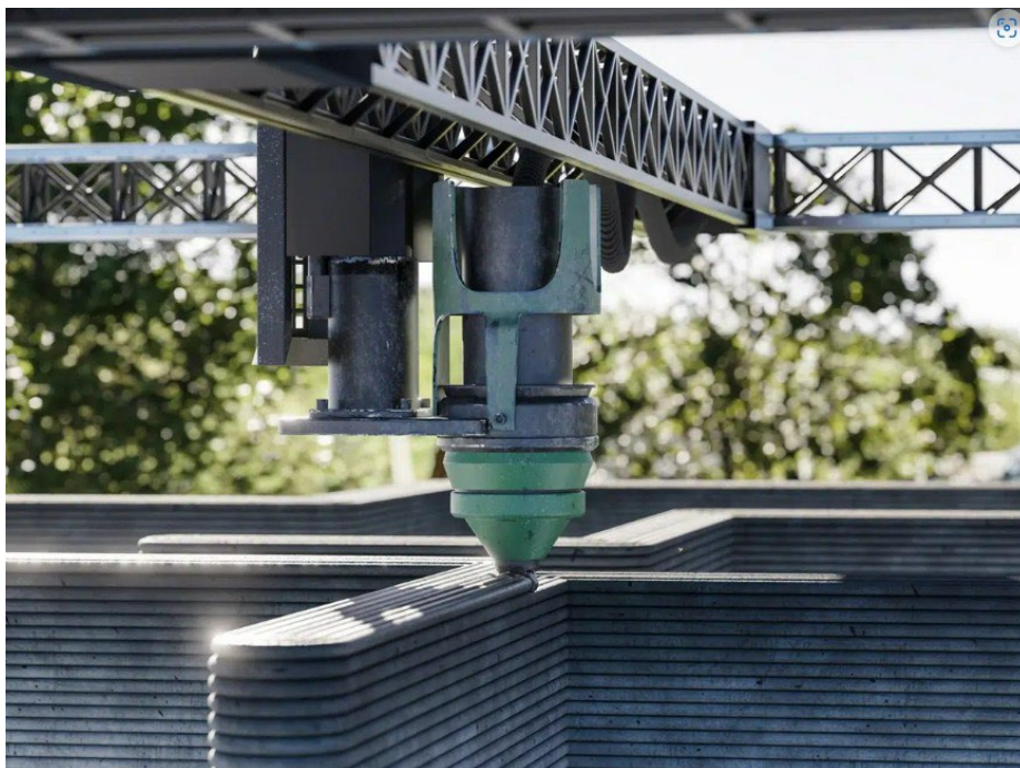
Figure 1. 3D-printed construction can reduce construction time and material waste while complementing traditional homebuilding.
