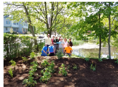
Rain garden construction showcase on the corner of Pond View Condo property, which abuts Butler's Pond.
