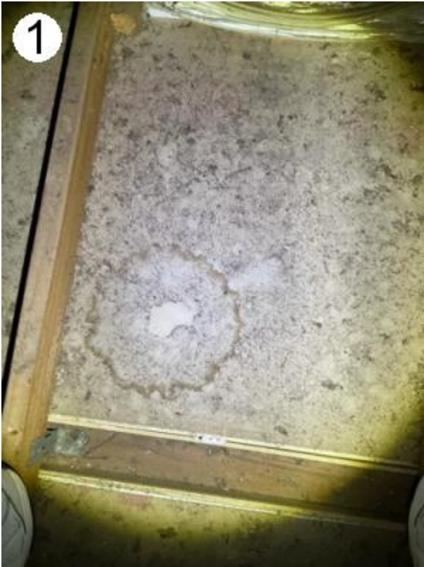
#1. Showing example of the moisture stains
