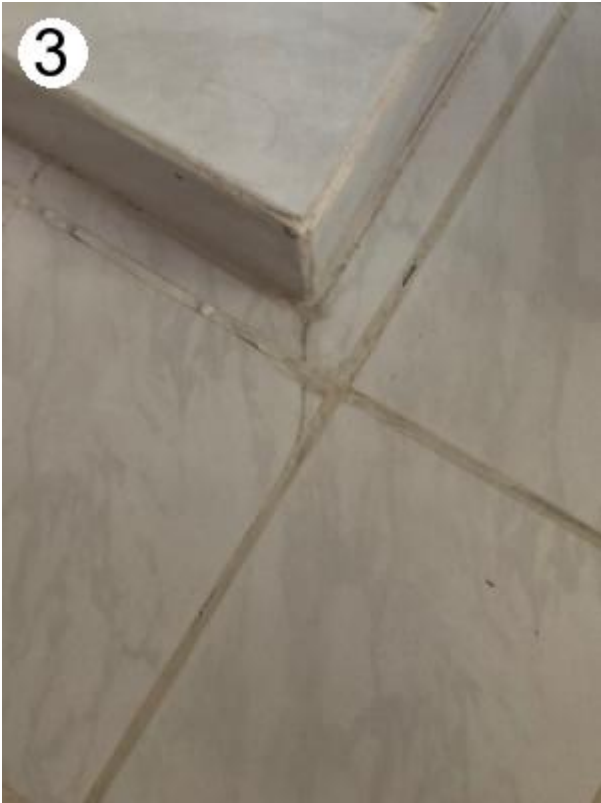
#3. Showing example of cracked tiles
