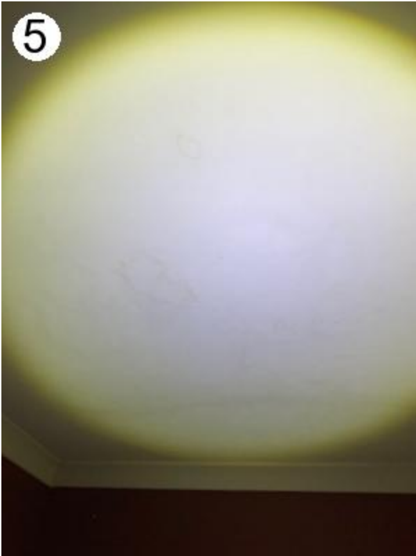
#5. Showing example of the stains
