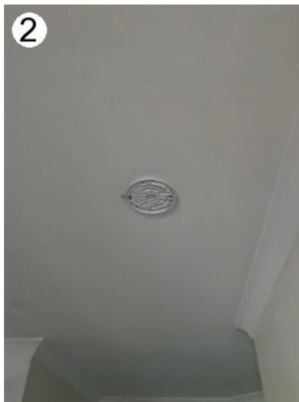
#2. Showing disconnected smoke alarm
