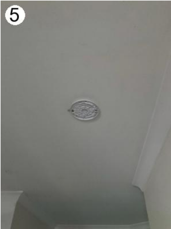
#5. Showing disconnected smoke alarm
