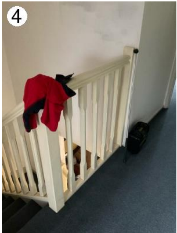
#4. Showing insufficient balustrades
