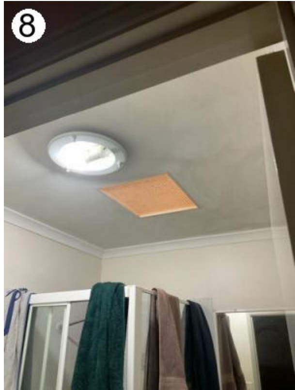
#8. Showing no exhaust fan
