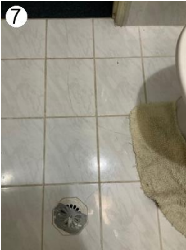
#7. Showing example of the cracked tiles
