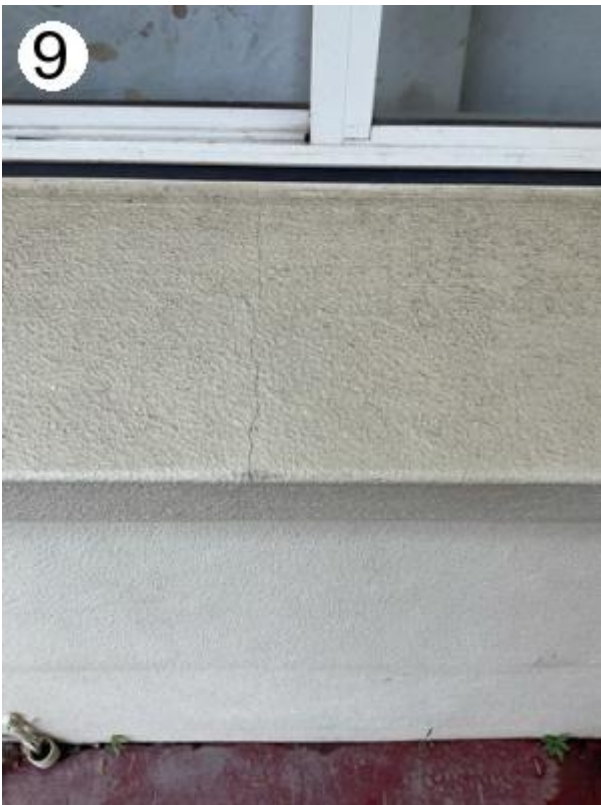
#9. Showing example of minor external wall cracks
