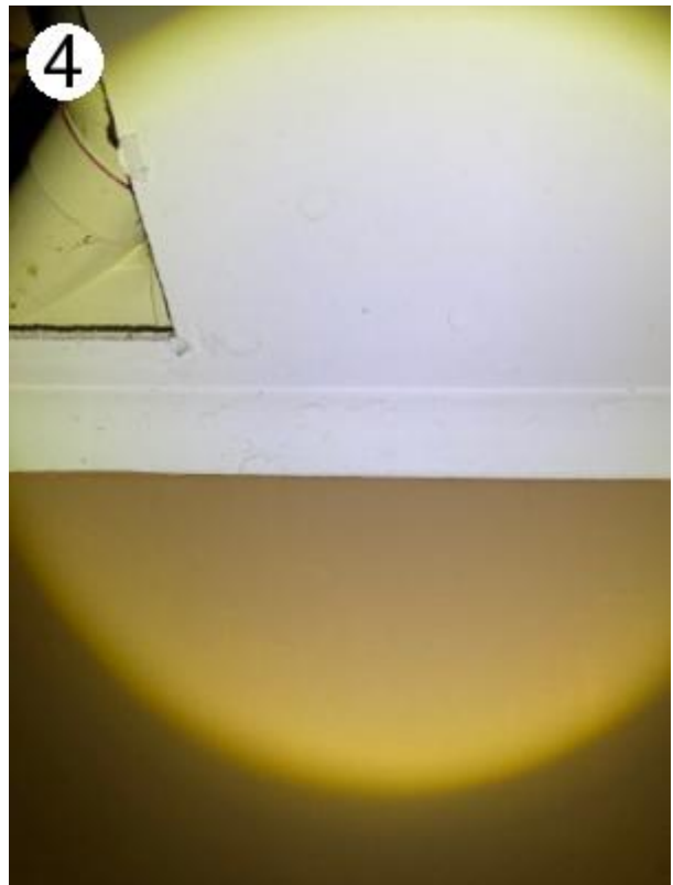
#4. Showing example of the stains
