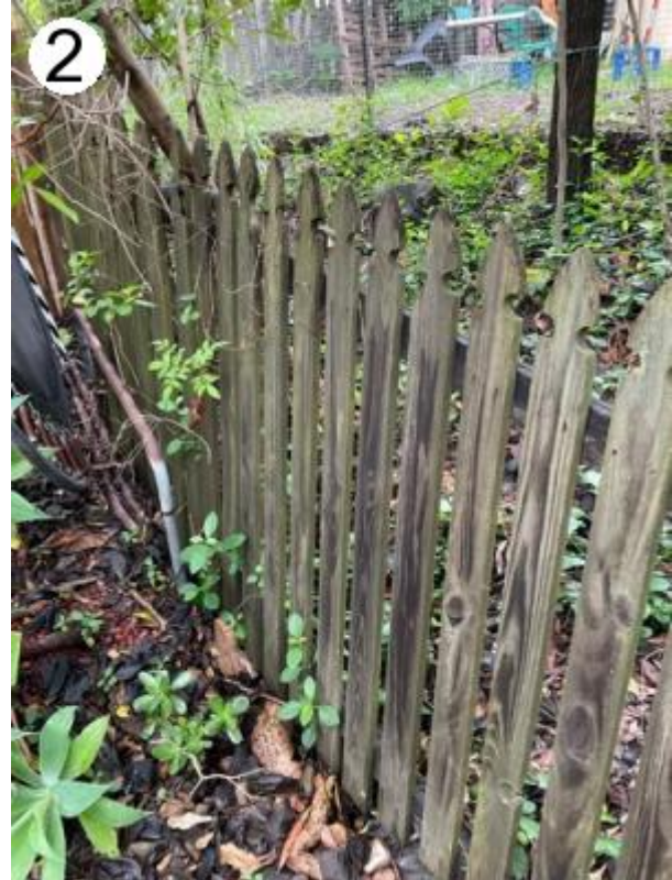
#2. Showing example of the rot and leaning fences
