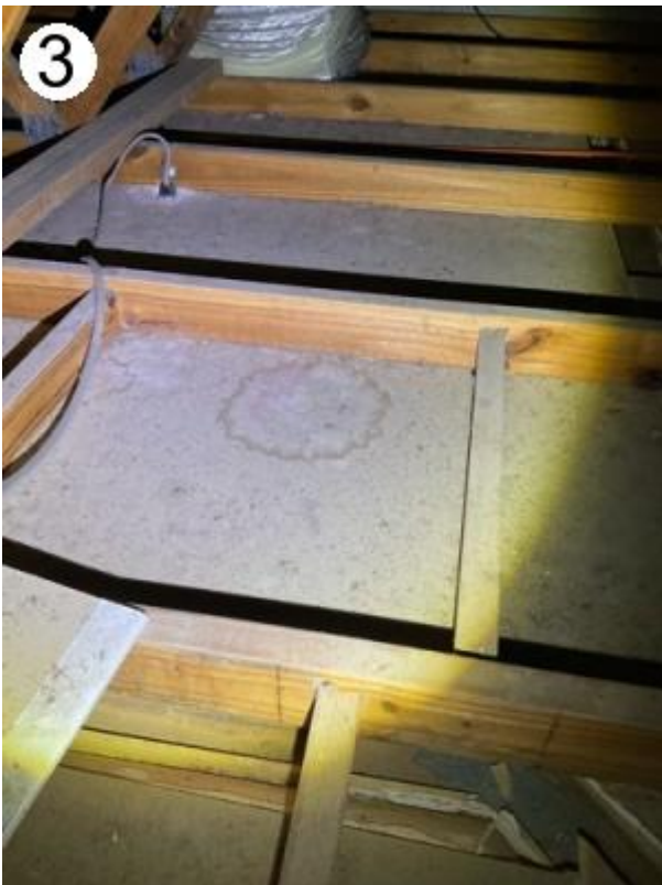
#3. Showing example of the moisture stains
