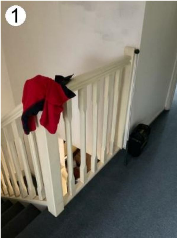
#1. Showing insufficient balustrades
