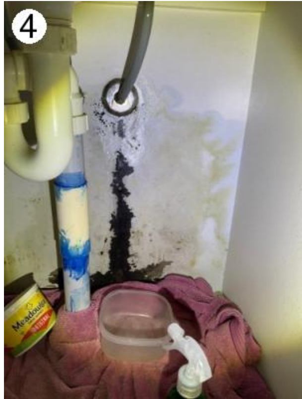
#4. Showing vanity moisture
