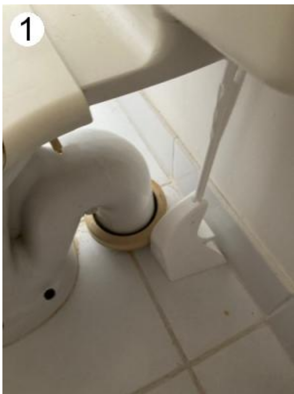
#1. Showing leaking toilet
