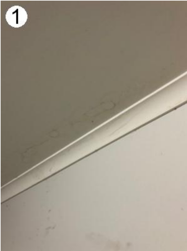
#1. Showing example of the stains
