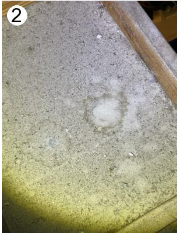
#2. Showing example of the moisture stains
