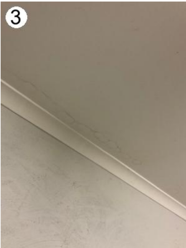
#3. Showing example of the stains
