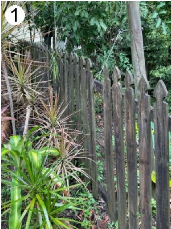
#1. Showing example of the rot
