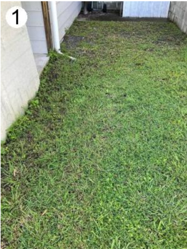
#1. Showing example of poor surface drainage
