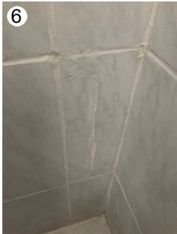
#6. Showing example of the cracked tiles
