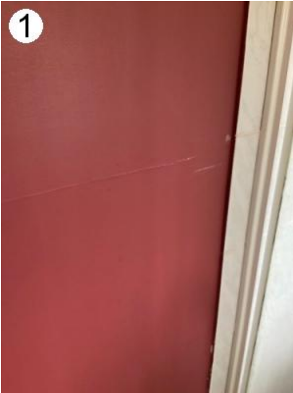
#1. Showing the cracks
