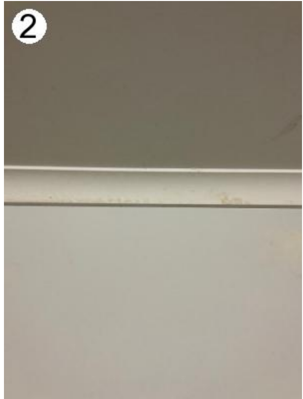
#2. Showing example of the stains
