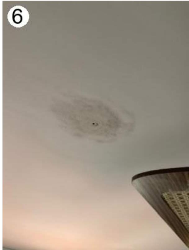
#6. Showing example of the stains
