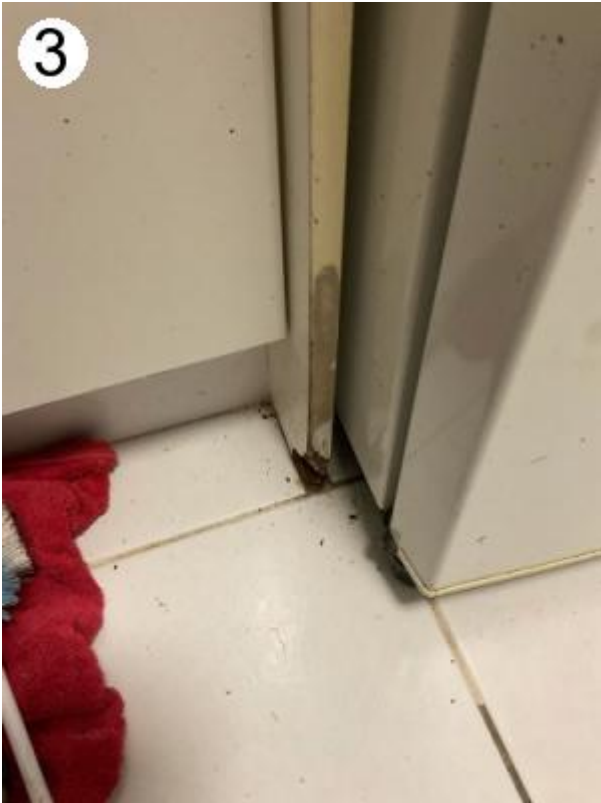
#3. Showing example of the cabinets
