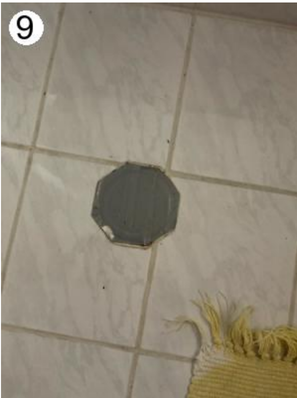
#9. Showing the floor waste
