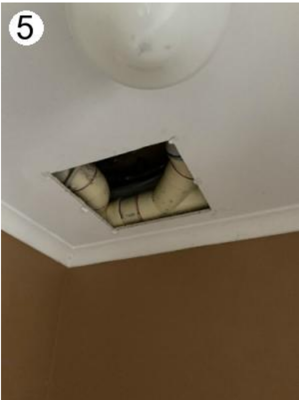
#5. Showing hole in ceiling
