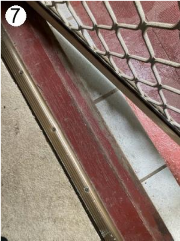
#7. Showing example of exposed weathered timbers
