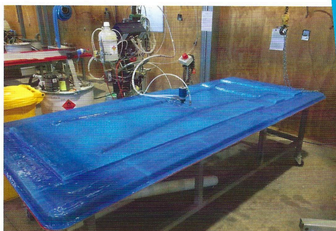
Deck section under-going the resin injection process using the latest silicone bagging technology.
