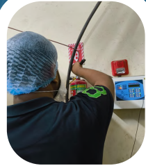
Fire Extinguisher Service
