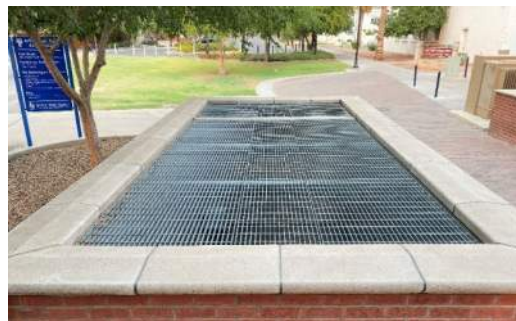
Figure 2: Exterior Mechanical Shaft Metal Louver
