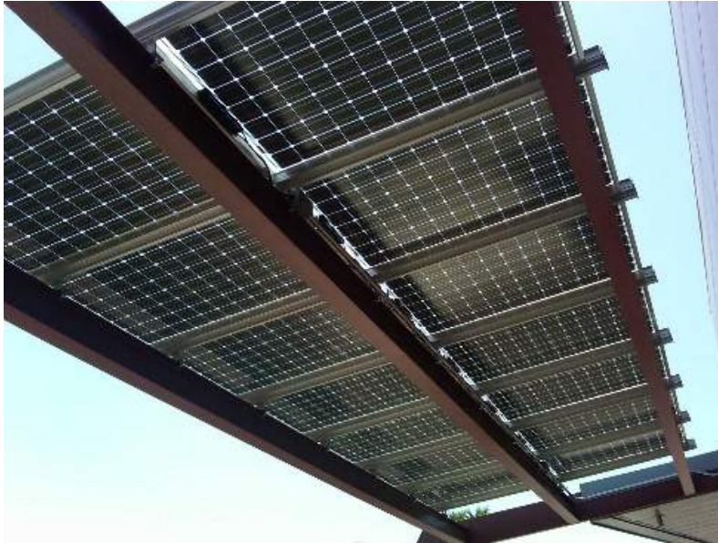
Figure 20: Solar Photovoltaic (PV) System
