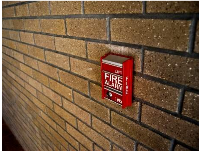
Figure 22: Fire Alarm System
