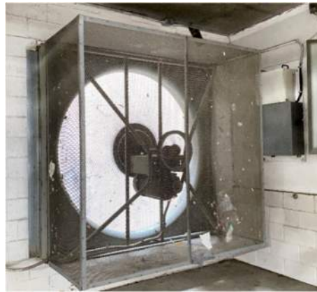
Figure 1: Sidewall Exhaust Fan
