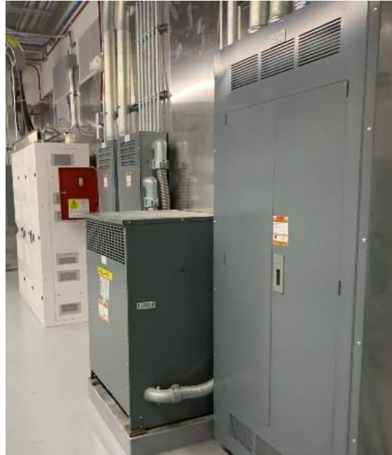
Figure 16: Switchboards, Panelboards, and Low-Voltage Transformers
