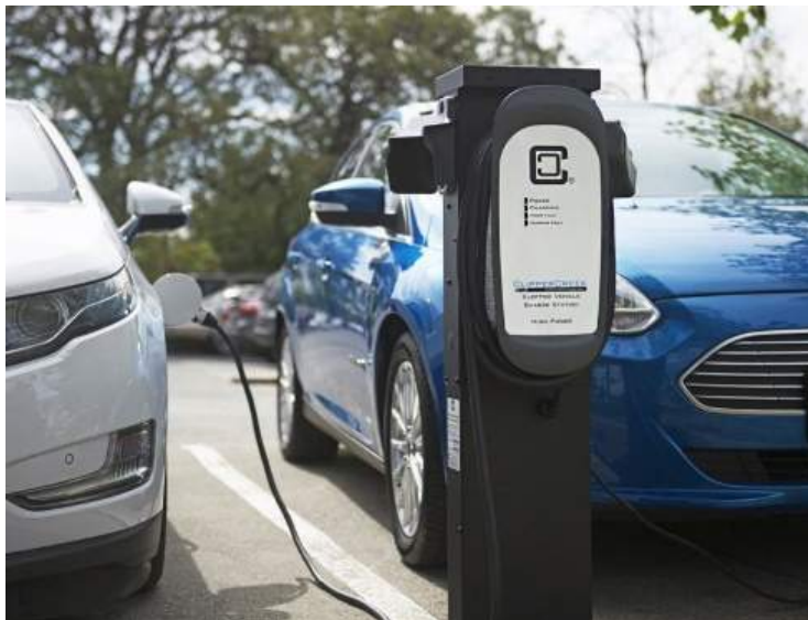
Figure 21: Electric Vehicle (EV) Charging Station
