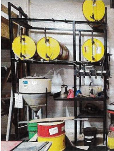
Maintenance Oil Storage
