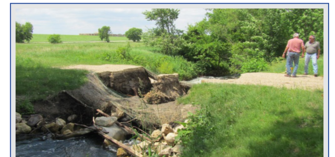
2014 Flood Damage Pictured is a culvert that was blow-out along the outlet channel last summer. Flood details from the PL/SLWD inside.
