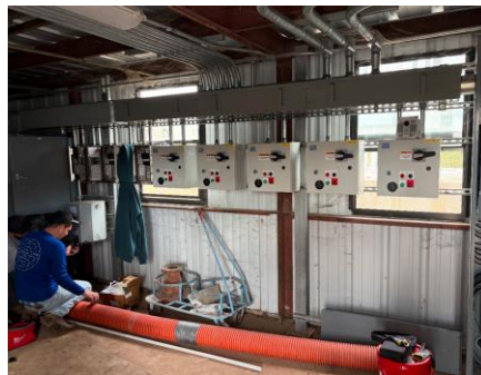
New MCC panels
