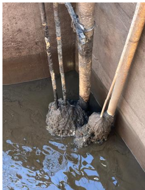
Flushables in sewer plant
