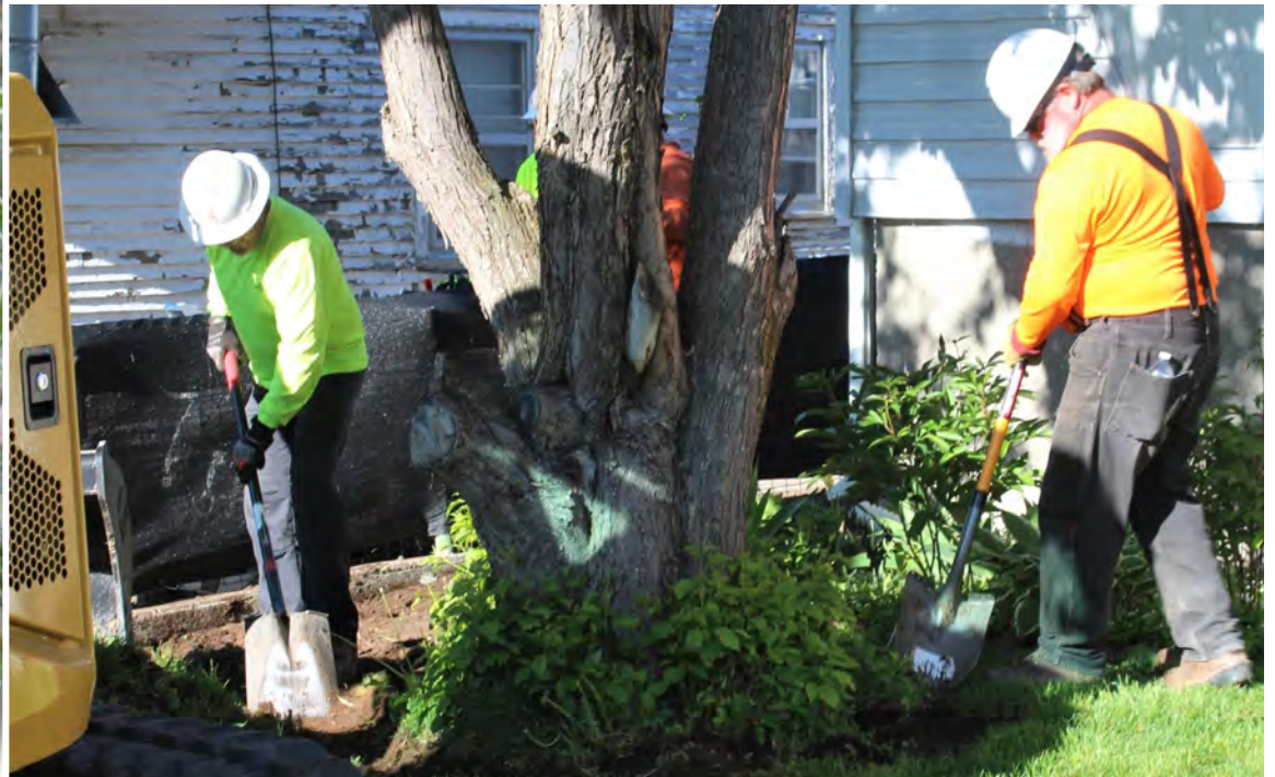
Environmental mitigation crews overseen by the U.S. Environmental Protection Agency have begun work in Black Eagle removing soils contaminated with lead and arsenic.
