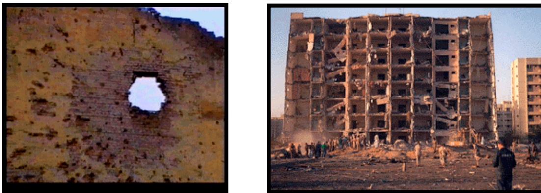
Figure 7-19. Examples of penetration and damage to buildings.
