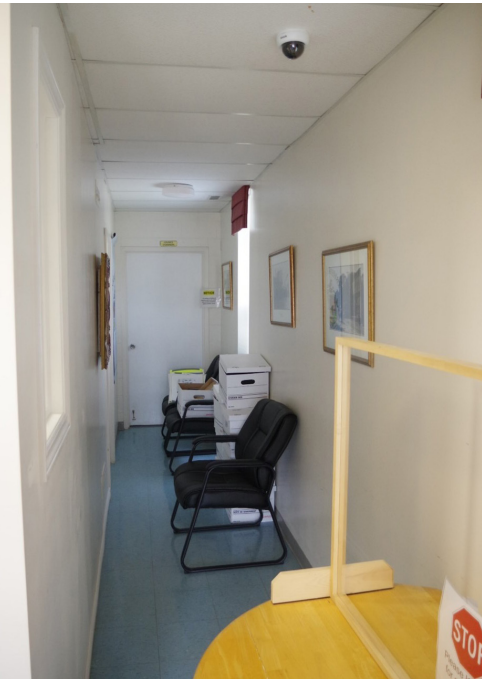
IMG 1.11 - Hallway space used as temporary overflow space, blocking safe travel for building users and not appropriate for barrier free access.
