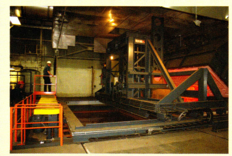
Complete Tip-up Furnace System with manipulator.
