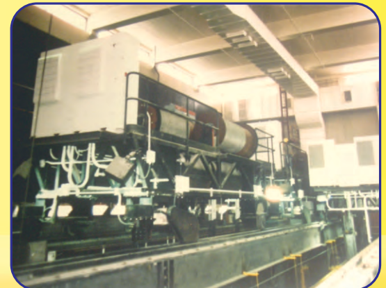
THE CAF-Cable Operated Bar Screen
