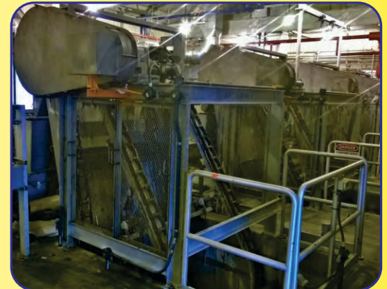
Catenary Bar Screen
