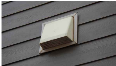
Exhaust Hood Vent
