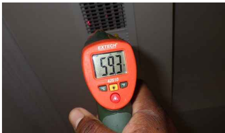
Room Supply Vents
