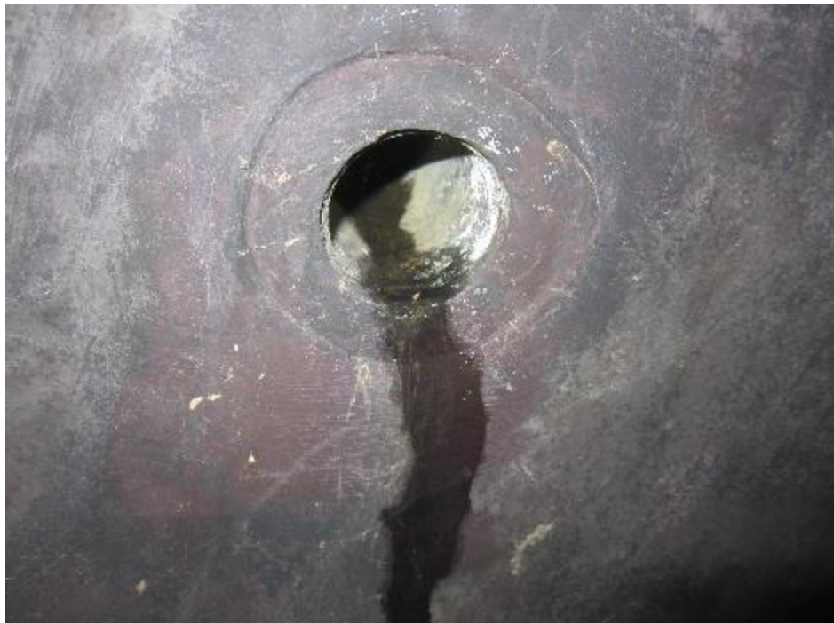
Figure 19 Bottom Through Hull
