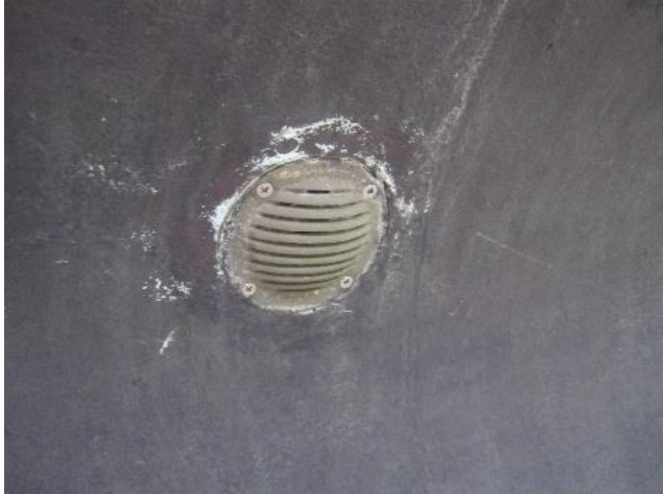
Figure 16 Bottom Through Hull
