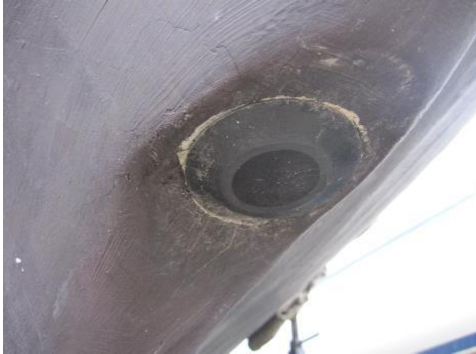
Figure 12 Bottom Through Hull
