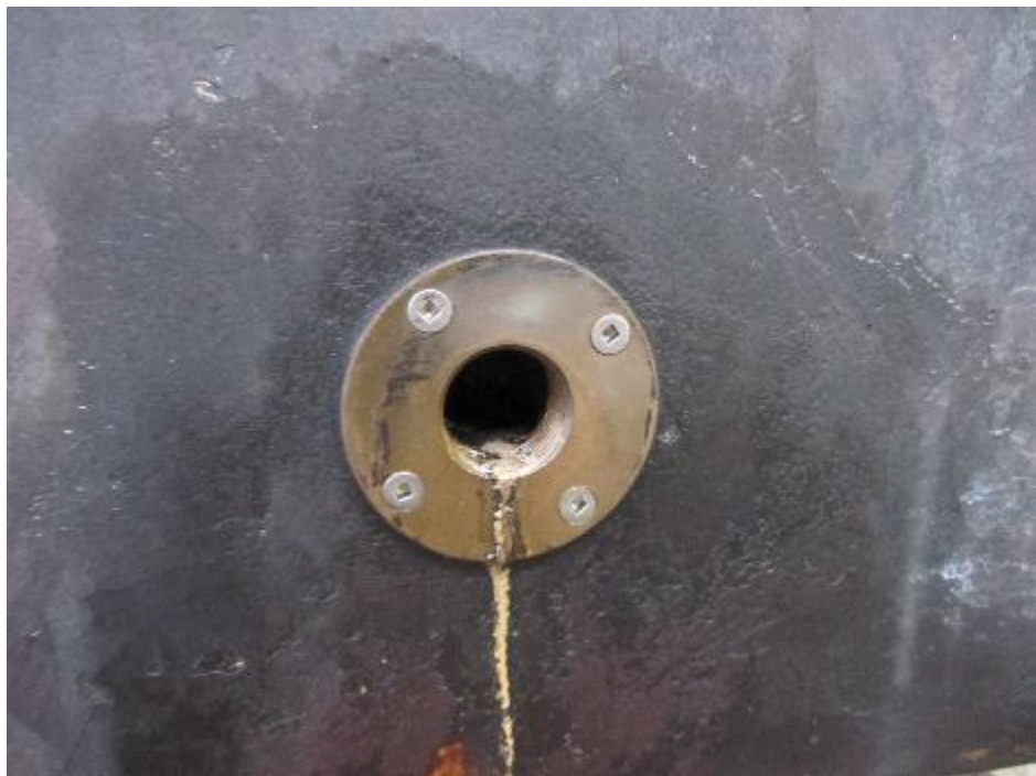
Figure 17 Bottom Through Hull
