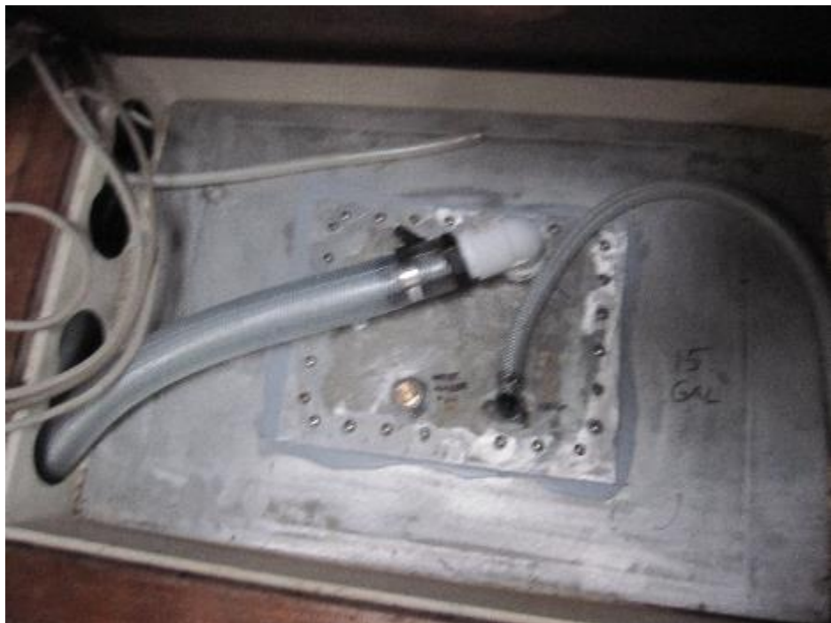
Figure 119 Hot Water Tank
