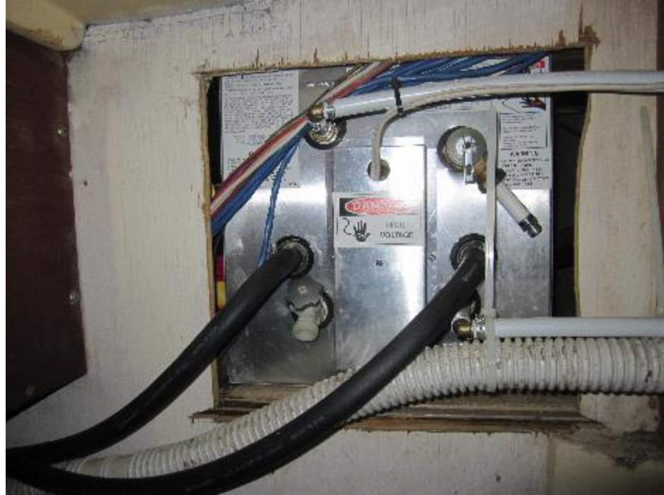
Figure 116 Hot Water Tank
