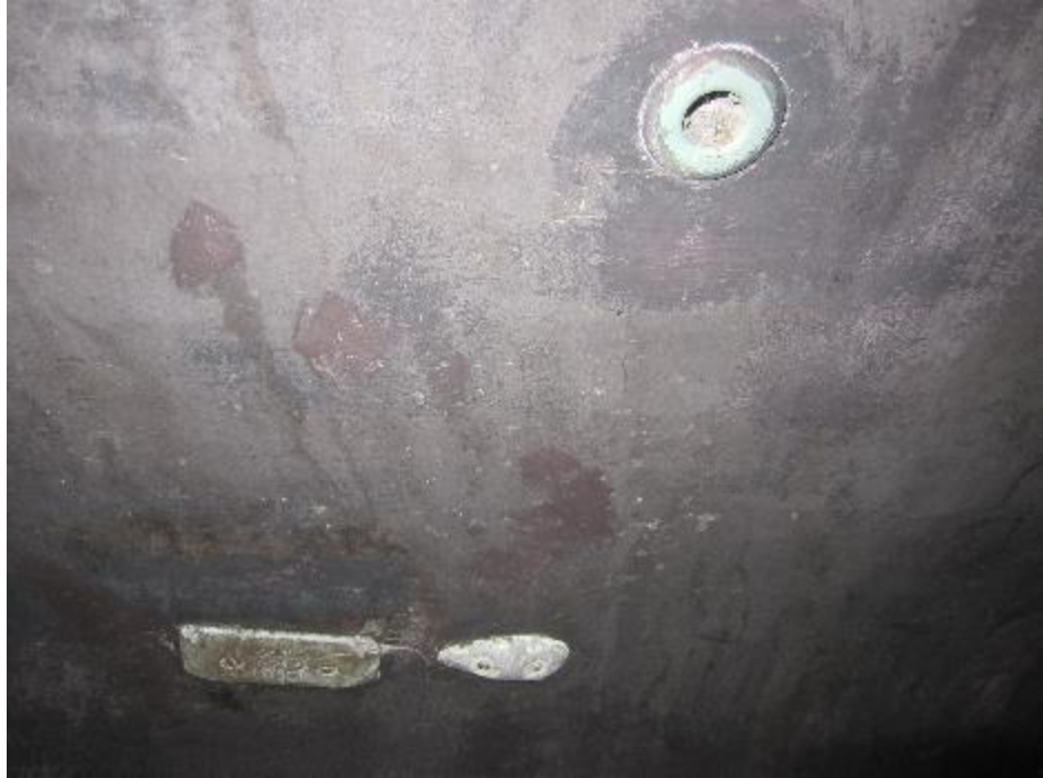
Figure 14 Bottom Through Hull
