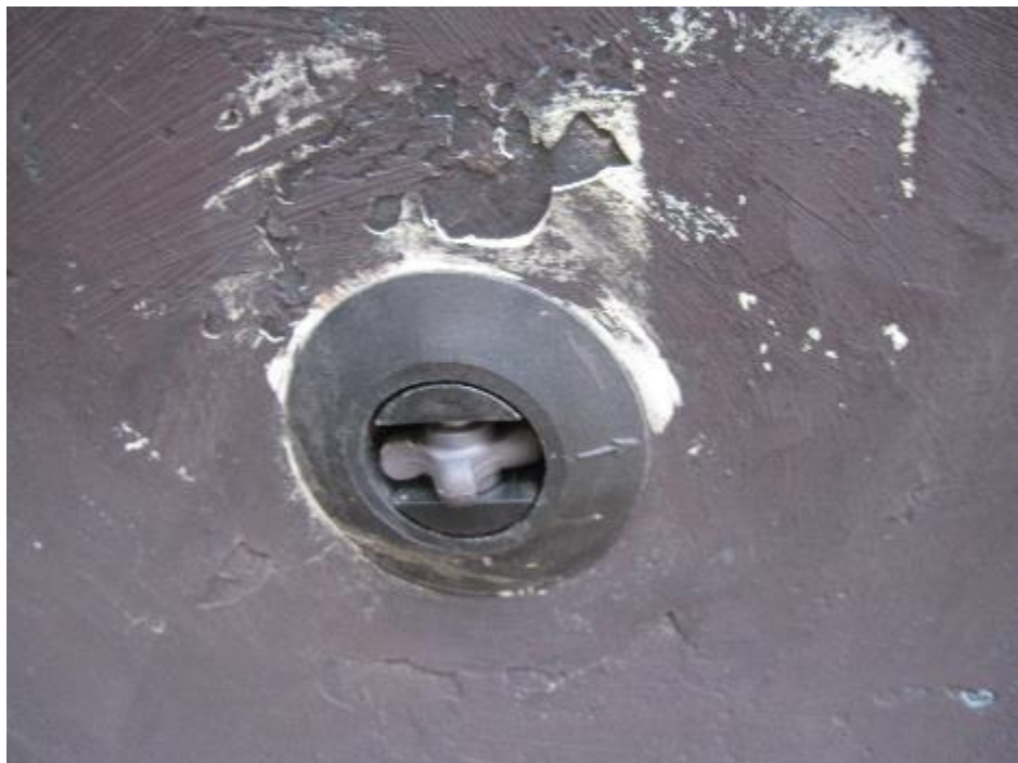
Figure 13 Bottom Through Hull
