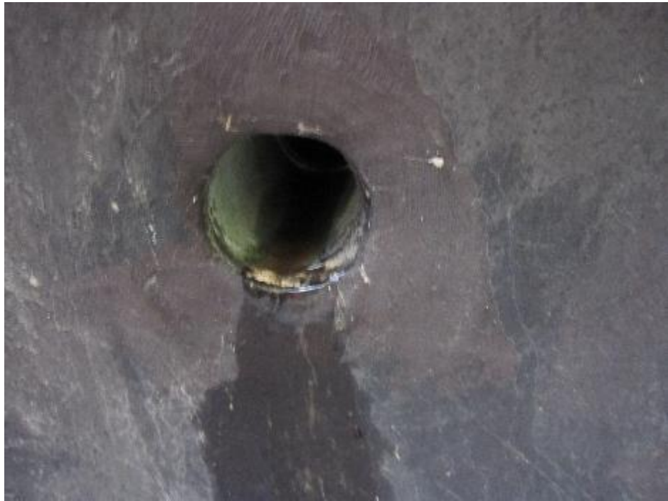
Figure 18 Bottom Through Hull
