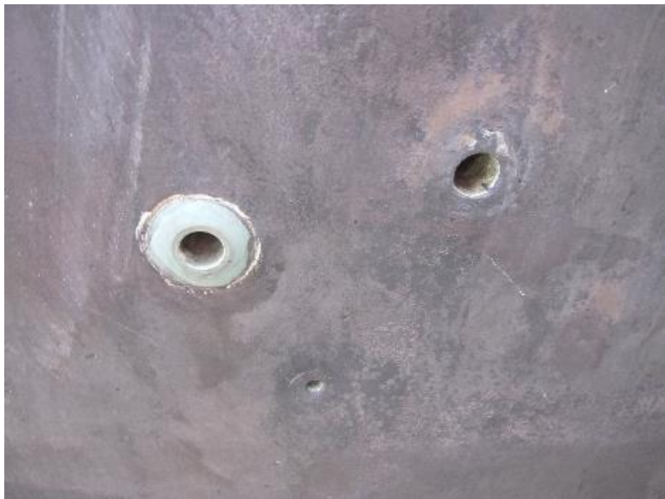
Figure 15 Bottom Through Hull
