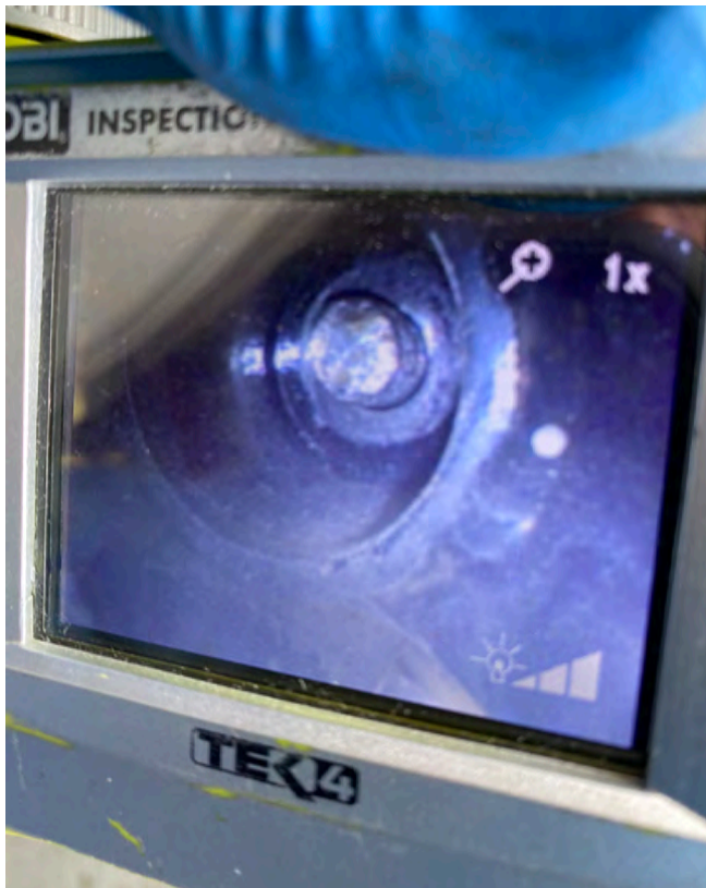
Bolt inspection missing nut.
