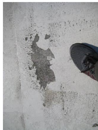
Coating separating from the roofing system.
