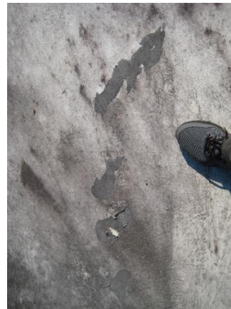
Coating separating from the roofing system.
