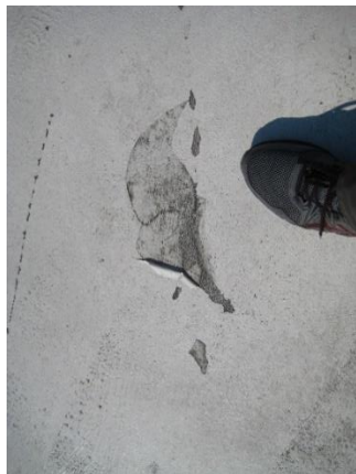
Coating separating from the roofing system.
