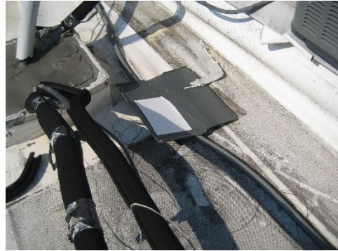
A/C pipig and debris.
