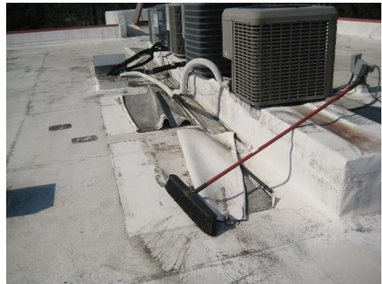
A/C system. Mat separating from the roofing system.
