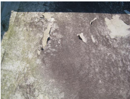
Coating separating from the roofing system.
