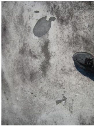
Coating separating from the roofing system.
