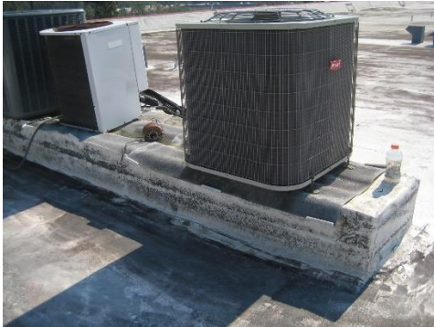
A/C system and debris.
