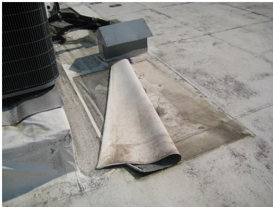
Roof mat separated from the roof system.
