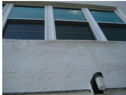
Cracks on windowsill.
