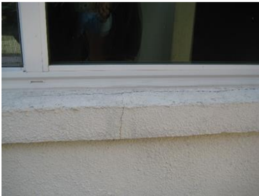
Minor cracks on windowsill.
