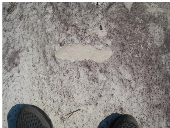
Coating separating from the roofing system.
