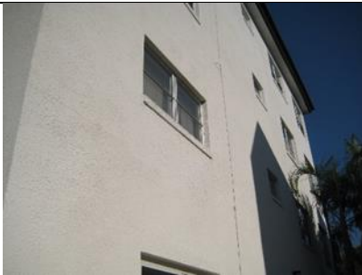
Typical exterior with cracks.
