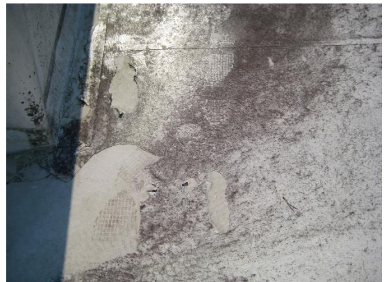
Coating separating from the roofing system.
