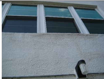
Typical exterior with cracks.
