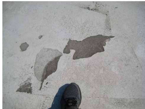
Coating separating from the roofing system.
