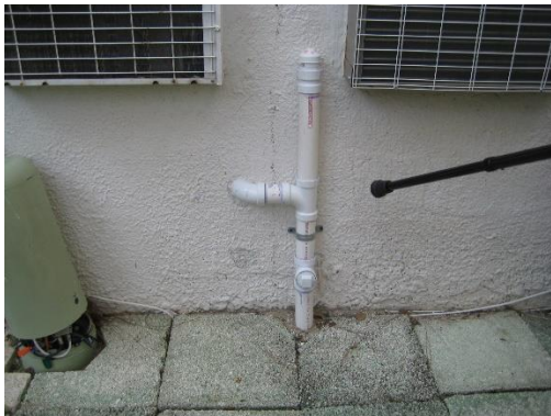
PVC Sewer line.
