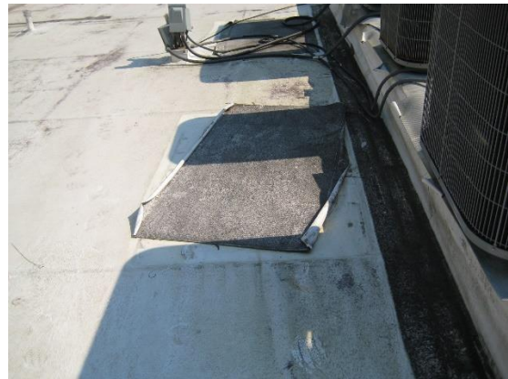
Roof mat separated from the roof system.
