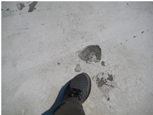
Coating separating from the roofing system.
