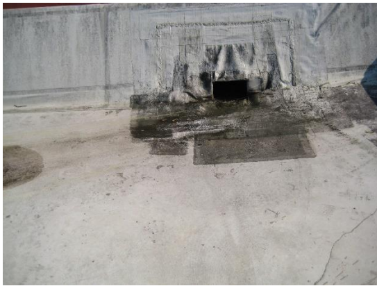
Drain to gutter; no screen.
