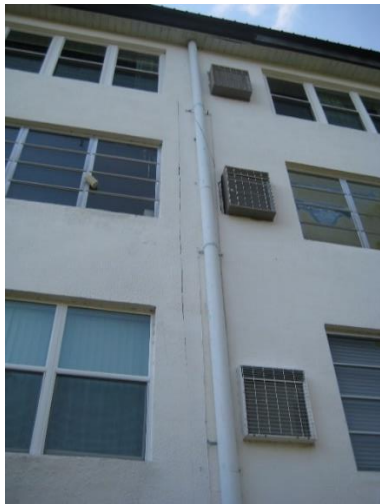
Openings around air conditioners.
