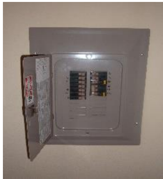
Example of an Electrical
