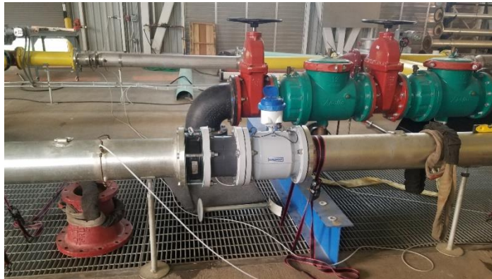
Figure 4 - Krohne WF flow meter 1 diameter downstream of a check valve
