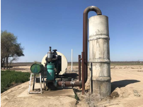
Figure 2 - Meter installed less than 2 diameters upstream of 90° bend
