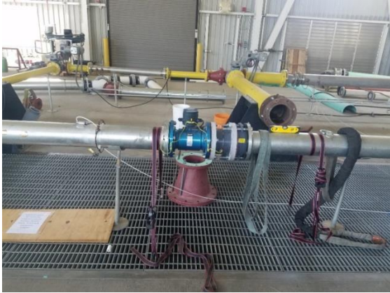
Figure 7 - Bermad Euromag flow meter 1-diameter upstream of a check valve
