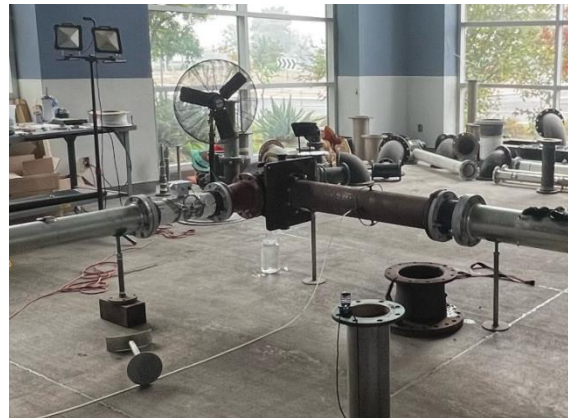
Figure 6 - McCrometer flow meter 1-diameter downstream of 90 bend
