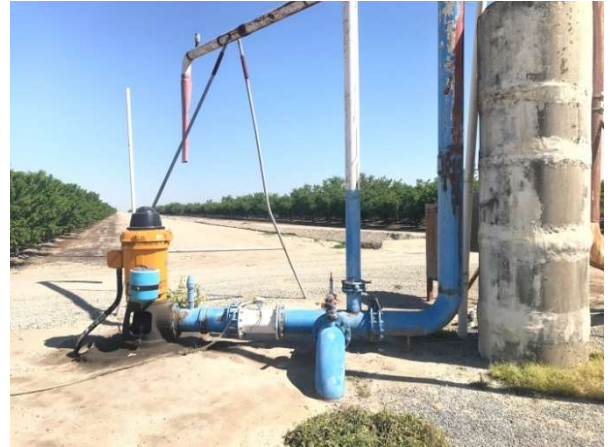
Figure 3 - Meter installed 2.5 diameters downstream of a pump discharge
