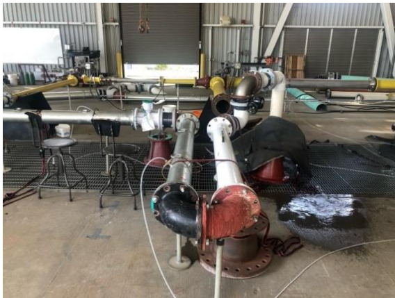
Figure 5 - Seametrics AG3000 1-diameter upstream of 90 bend
