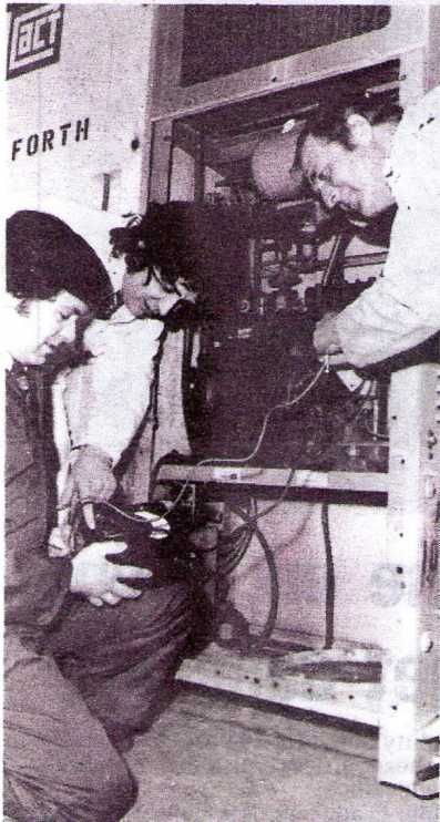
"It Ain't Half Hot Mum" — Refrigeration technicians at Seaforth inspect a refrigeration unit to make sure that everything is working perfectly. They are (left to right) E. Roberts, D. Heather and P. May.
