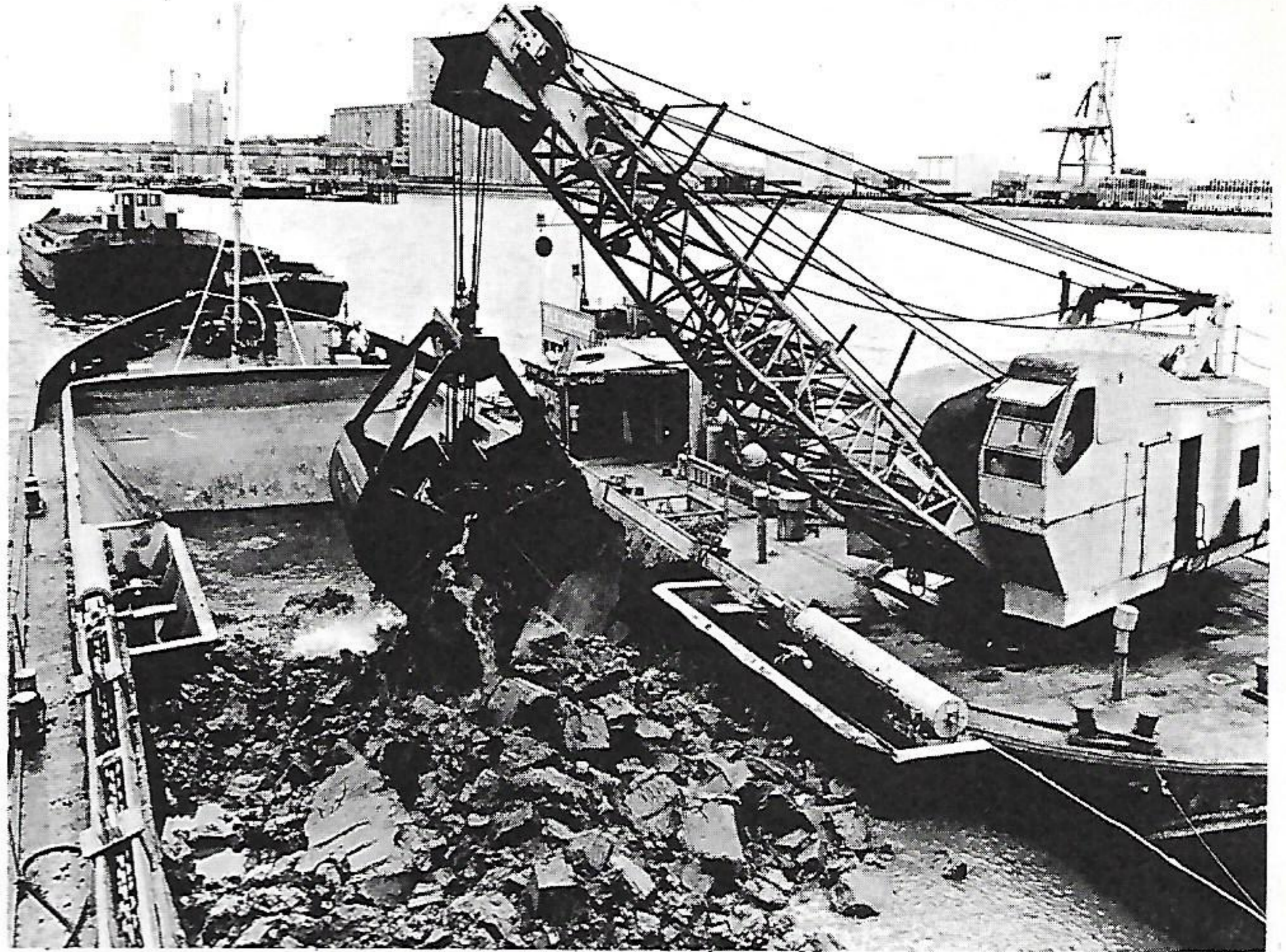
Reclamation of 25 acres for the new riverside container berth at Tilbury has begun. In the photograph the PLA grab dredger "George" is shown at work in Northfleet Hope removing the clay overlay from the river-bed to expose the gravel beneath, which will be used in the reclamation project. The Tilbury Grain Terminal is visible (upper left) and part of the multi-user container berths (upper right) are also pictured.
