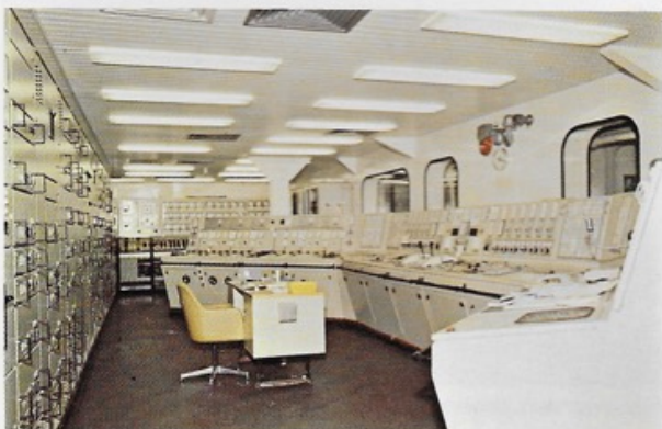
Fully automated control room.
