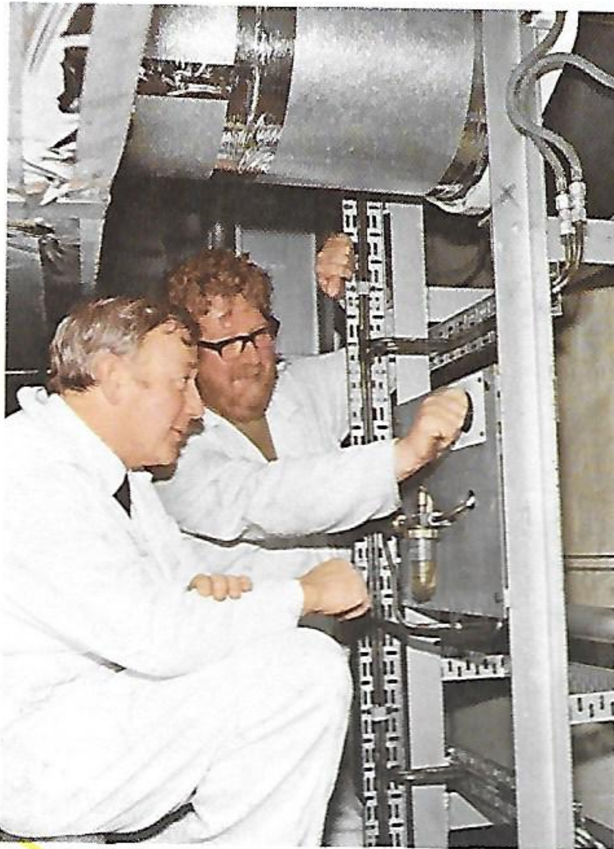
It's a long climb down but Capt. Leighton personally inspects refrigeration unit in the hold with Chief Engineer Ronnie Waugh.
