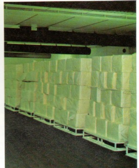
The bulk butter is then transferred into conditioning rooms for the temperature to be raised from -10^{\circ}\text{C} to between 0^{\circ}\text{C} and 2^{\circ}\text{C} . The warm air ducts can be seen in the ceiling.
