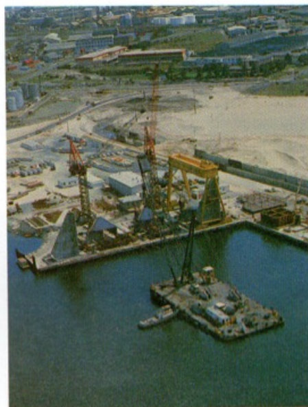
It took 19 years of research, dredging, reclamation and construction to carry out the programme and in this photograph, the Container Terminal, with six container berths, nears completion.
