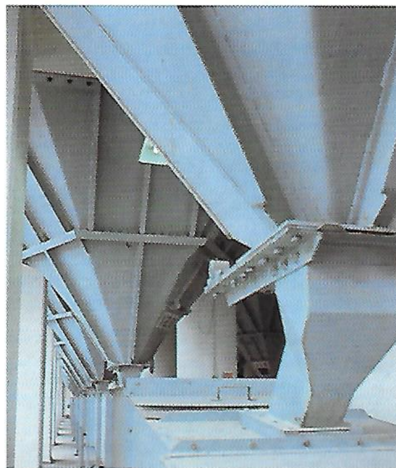
Partial view of the silo block at Wallingford with a capacity for storing 38,000 tonnes of malt and barley until needed.
