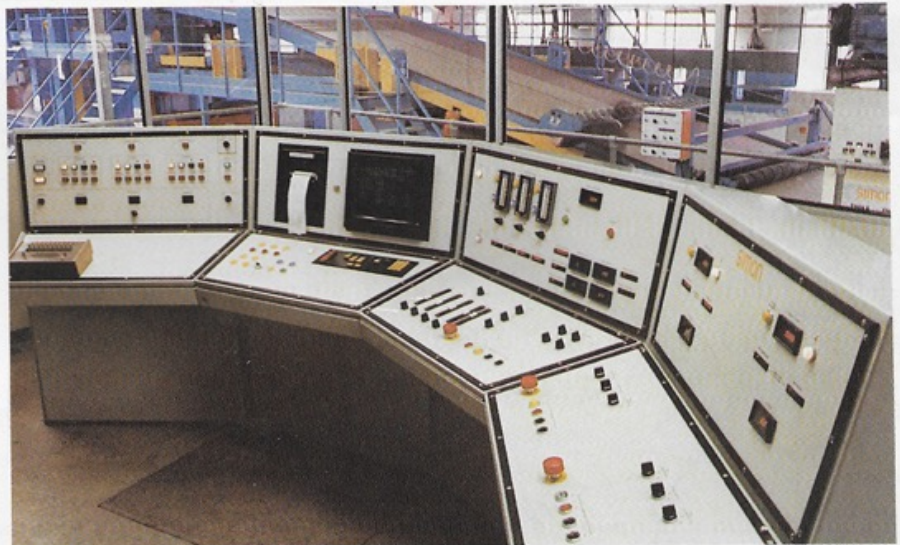
Simon Corrugator Central Control Desk from which the operation is controlled.
