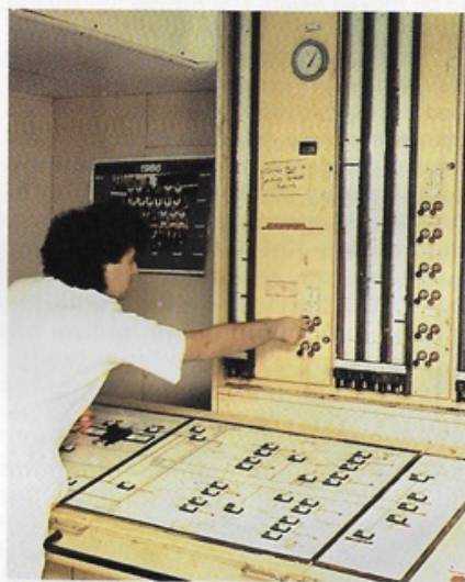
Partial view of the refrigeration control panel on Harrison Line's M.V. Author. At sea temperatures are carefully monitored and strictly controlled to ensure that the yucca arrives in prime condition.
