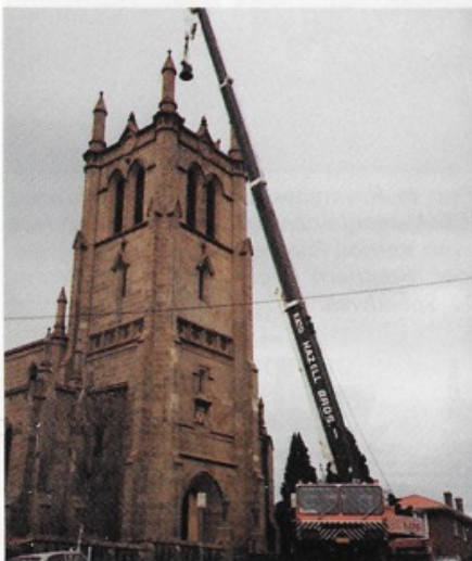
The "Fifth" bell is taken out of the top of the bell tower of Holy Trinity Church in Hobart prior to being loaded for shipment to the UK by ACT(A).
