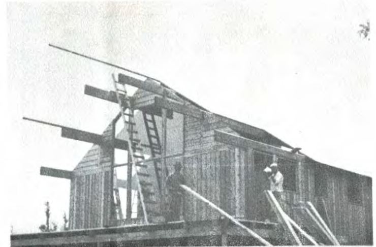
Under construction is the home of Mr. and Mrs. Ballard from Virginia.
