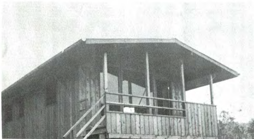
Nearing completion is the home of Mr. and Mrs. Piercy of Kailua-Kona.
