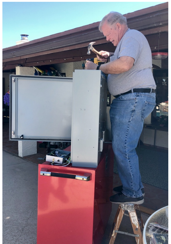
Don Stewart opens wiring ports on the new power supply cabinet with circuitry designed by John Mick.
