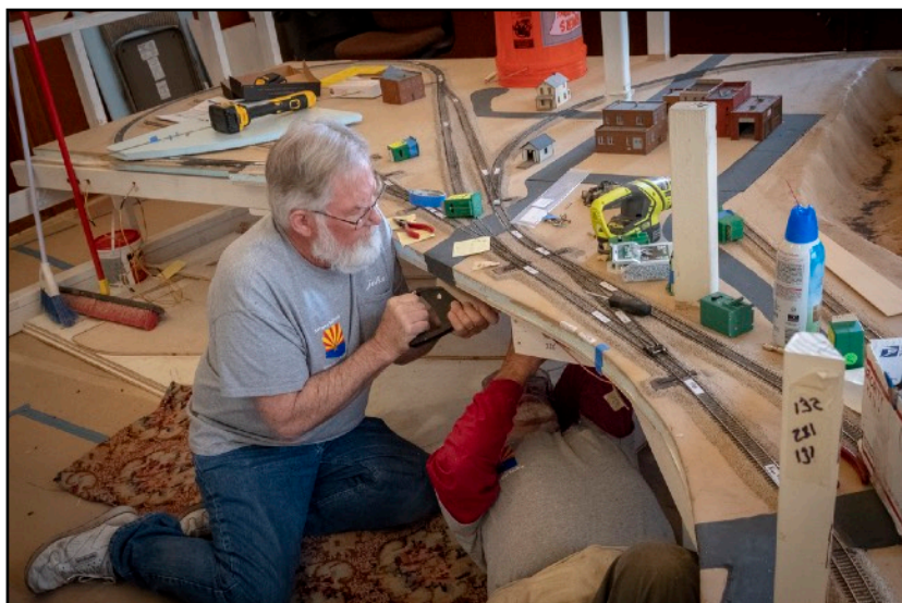
John Clark and Ray Rumble (under the layout ) have installed the majority of the Tortoise switch machines on the lower level. photo by Bob Bridges
