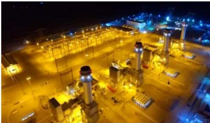
DHIQAR Combined Circulation Power Plant
