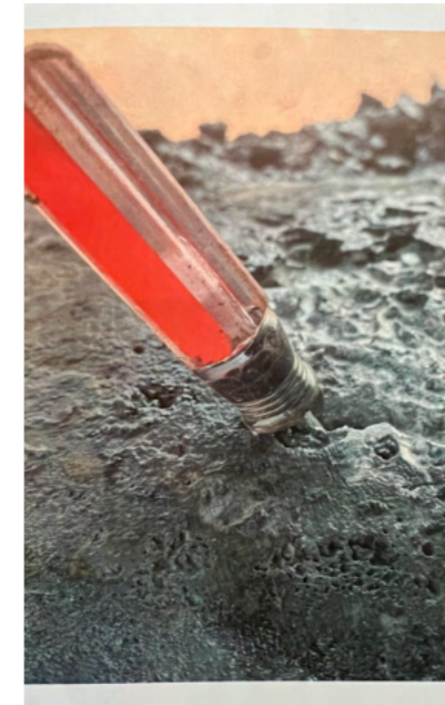
Screwdriver showcasing fire tube damage found with scanner
