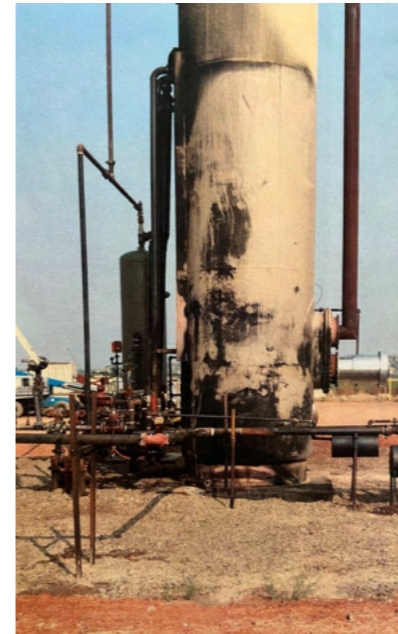
Commonplace heater-treater fire
