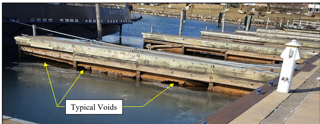
Figure 1: Typical Finger Pier Condition
