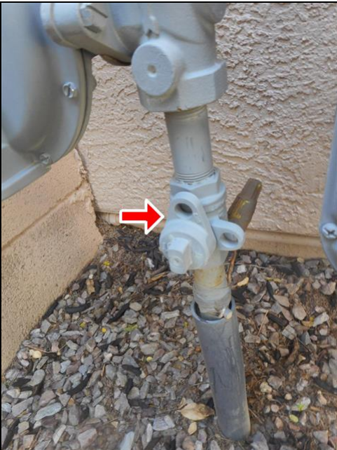
5.5 Item 1(Picture) Main fuel shut off
