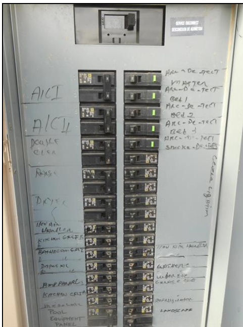
Electrical panel labeled breakers
