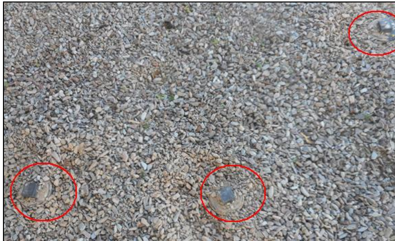
General shot of plumbing cleanouts in front
