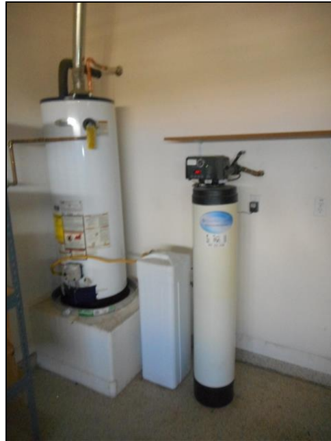
General shot of water heater and soft water systems
