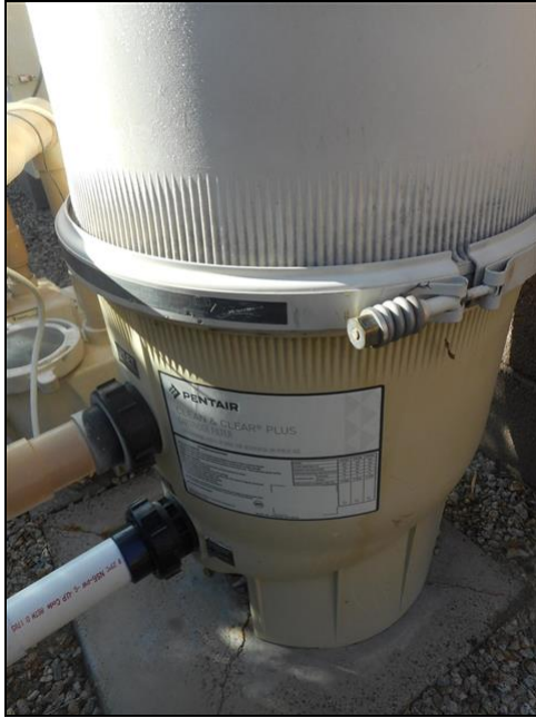
General shot of pool filter housing
