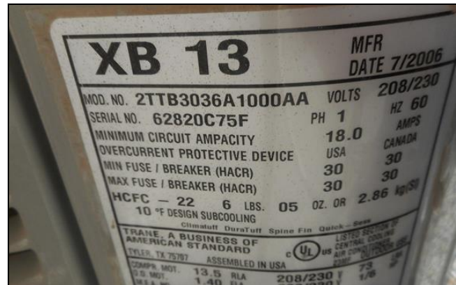
Data plate on HVAC compressor with smaller casing
