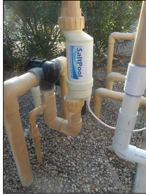
General shot of plumbing and valves
