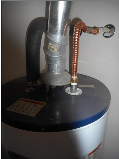
General shot of water heater connections
