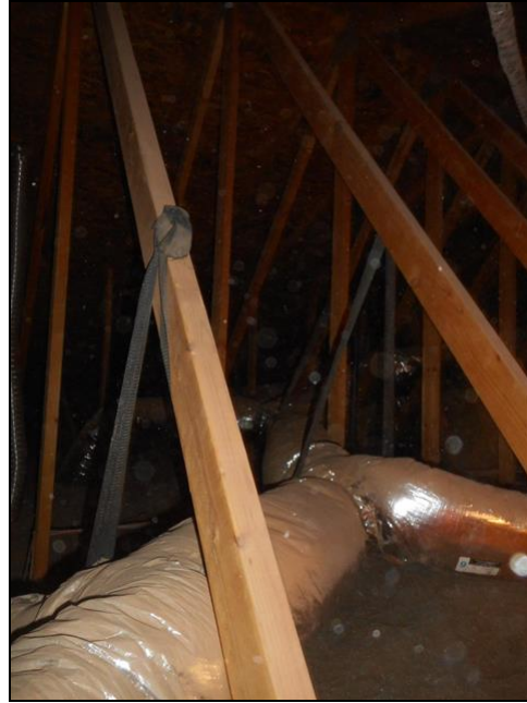
General shot of HVAC ducting and supports
