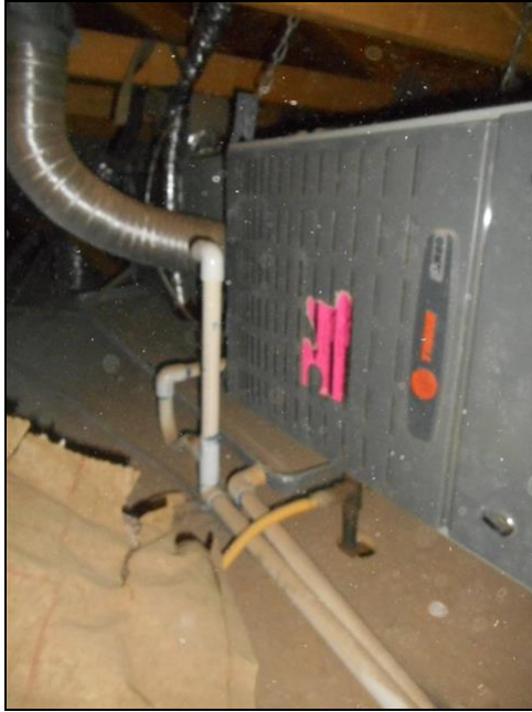
General shot of air handler above Master closet
