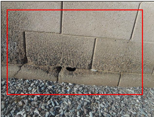
2.7 Item 4(Picture) Front of the house on the North adjacent to the driveway
