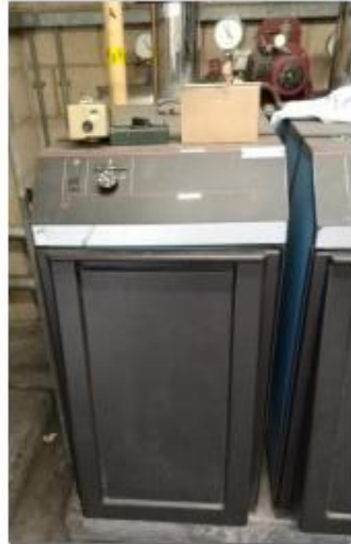
Aging gas fired boiler
