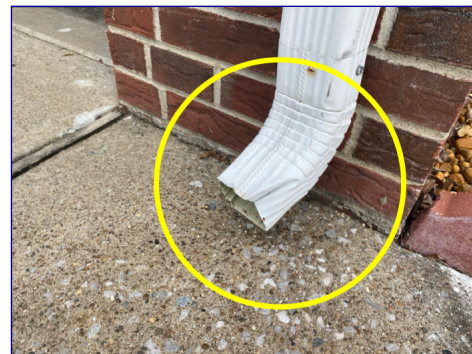
Damage, Recommend repair.
