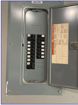
The electrical sub panel.
