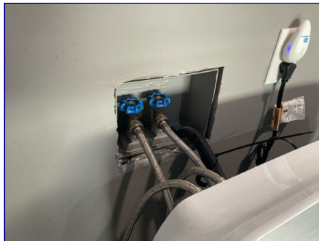
Laundry, washer hook-up view
