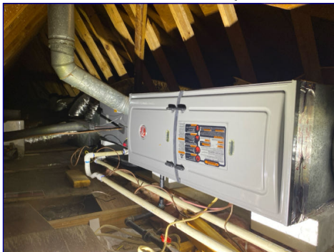
The furnace area
