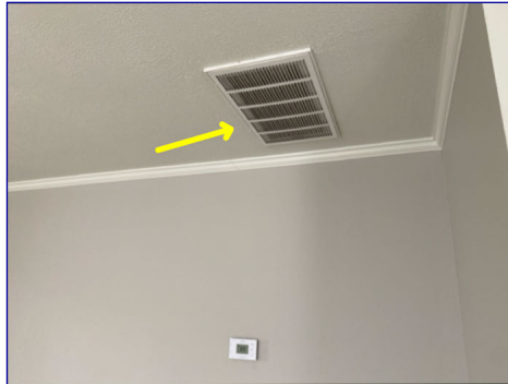
HVAC filter location.
