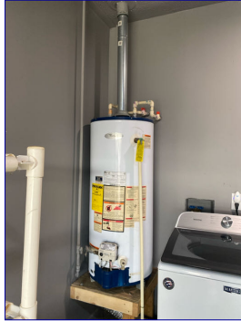
The Water Heater Area
