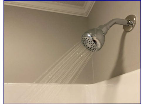
Shower water flow.
