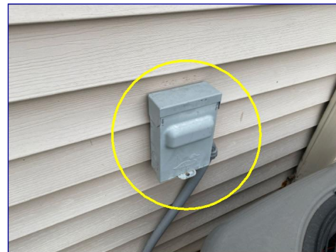
Local HVAC disconnect location
