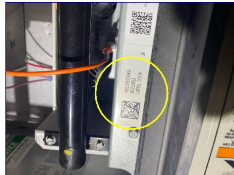
The furnace, data tag
