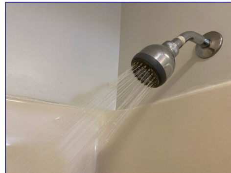
Shower water flow.
