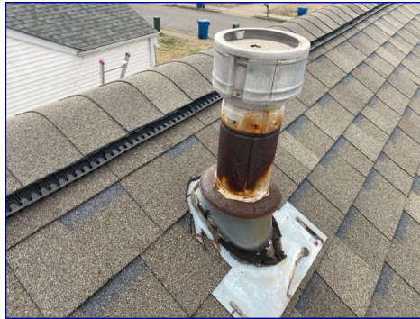
The HVAC vent is rusted. Recommend a licensed contractor replace the vent.
