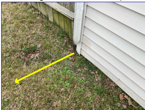
The downspout is missing. Recommend a licensed gutter contractor install a downspout and downspout extension.
