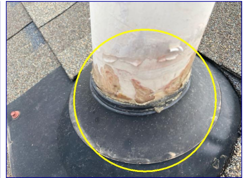
The plumbing vent needs to be caulked to prevent water intrusion. Recommend licensed roofing contractor repair.
