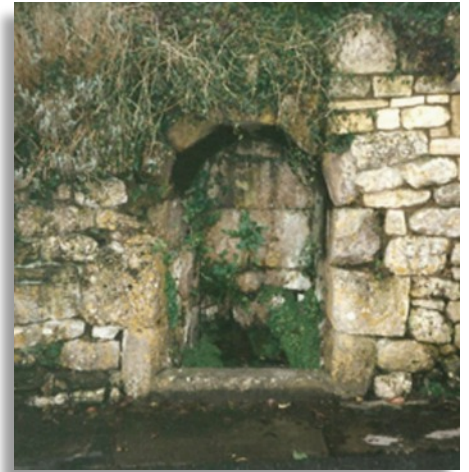
Lower Stoke trough in disrepair
