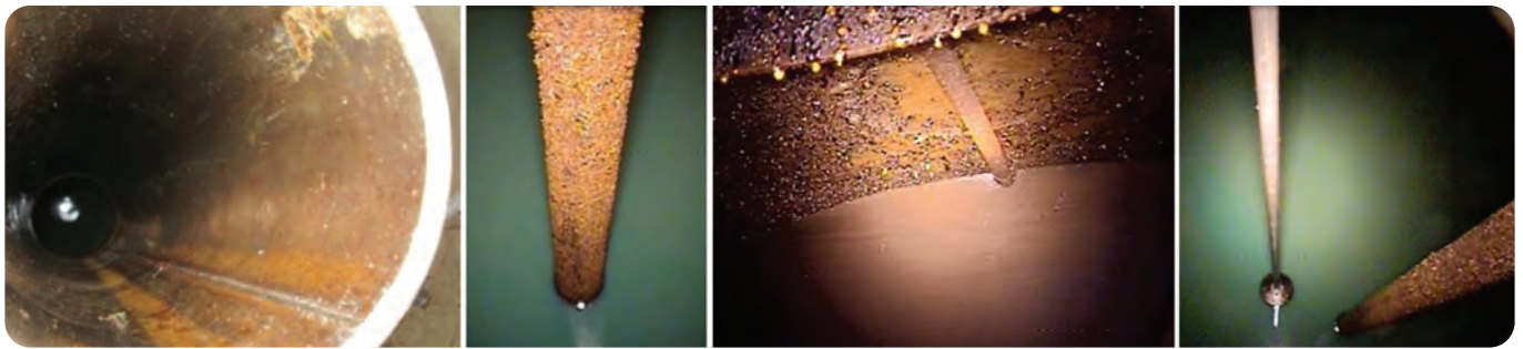
Figure 4. UST system with steel tank with severe metal corrosion (43-MD-ST: [installed 1992; age of filter unknown). From left: fill pipe opening; STP shaft; tank top showing manway; ATG probe and STP shaft. 3
