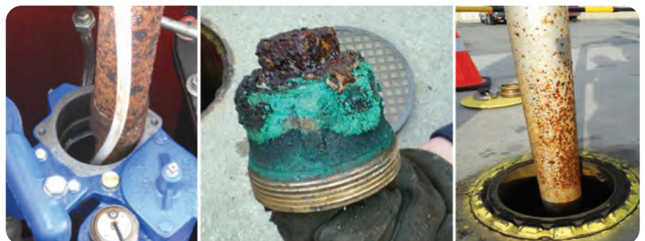
Figure 3. Corroded ULSD equipment: Corroded carbon steel submersible turbine pump (STP) shaft removed from pump housing, CA-1 (left); brass ball float extractor cage plug, NY-2 (middle); aluminium drop tube, NC-1 (right). 2
