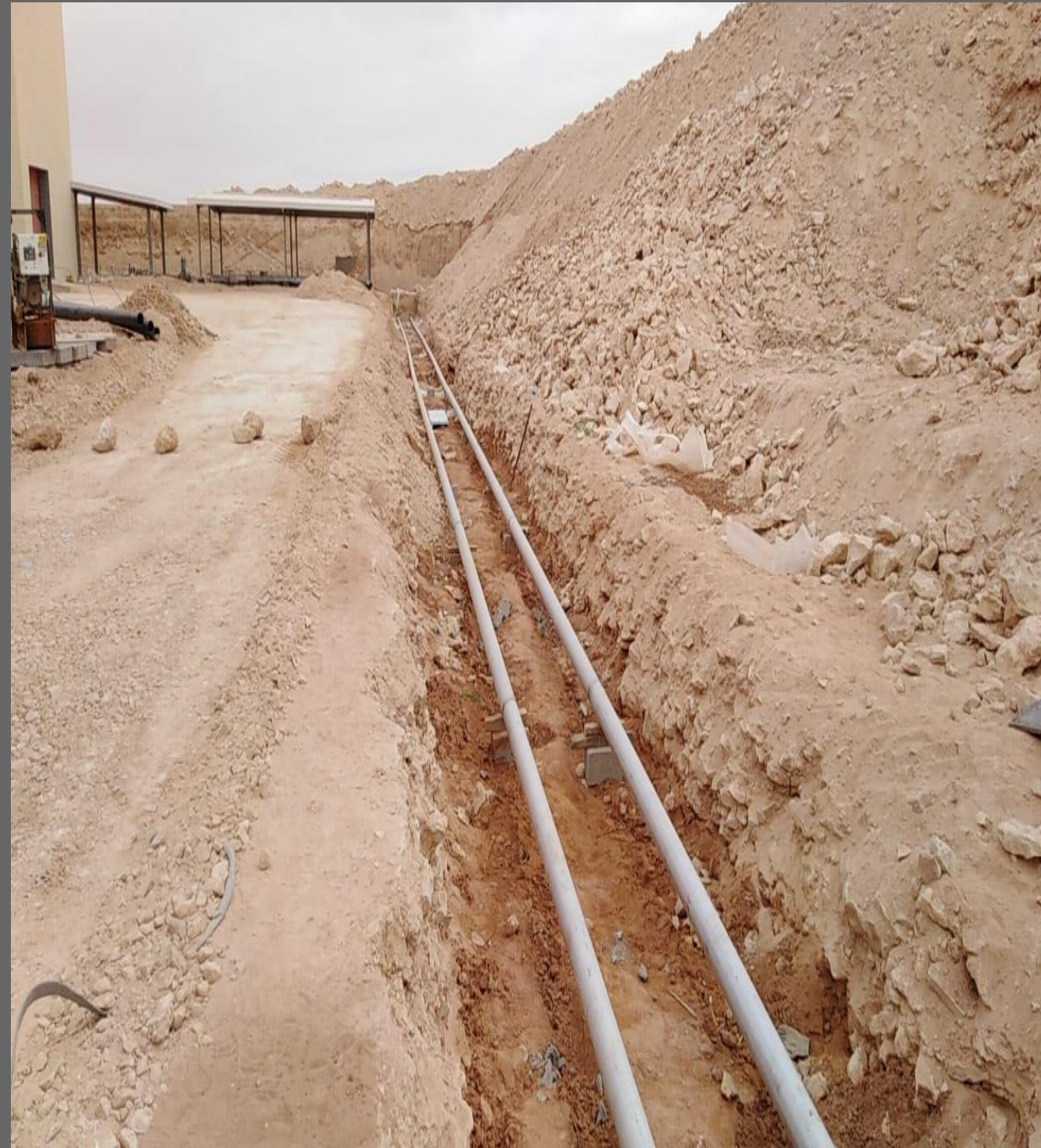
Industrial Network SS Pipe 6" underground
