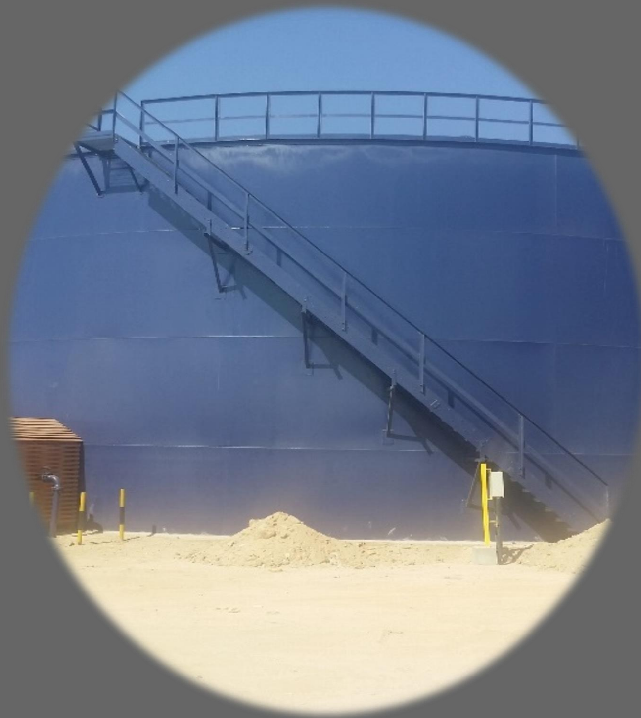
Steel Storage Tank 5,000m 3 Dia: 27.23m
