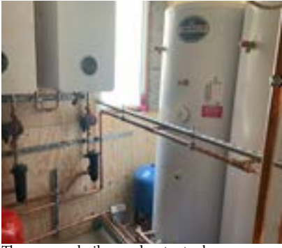
The new gas boilers and water tanks
