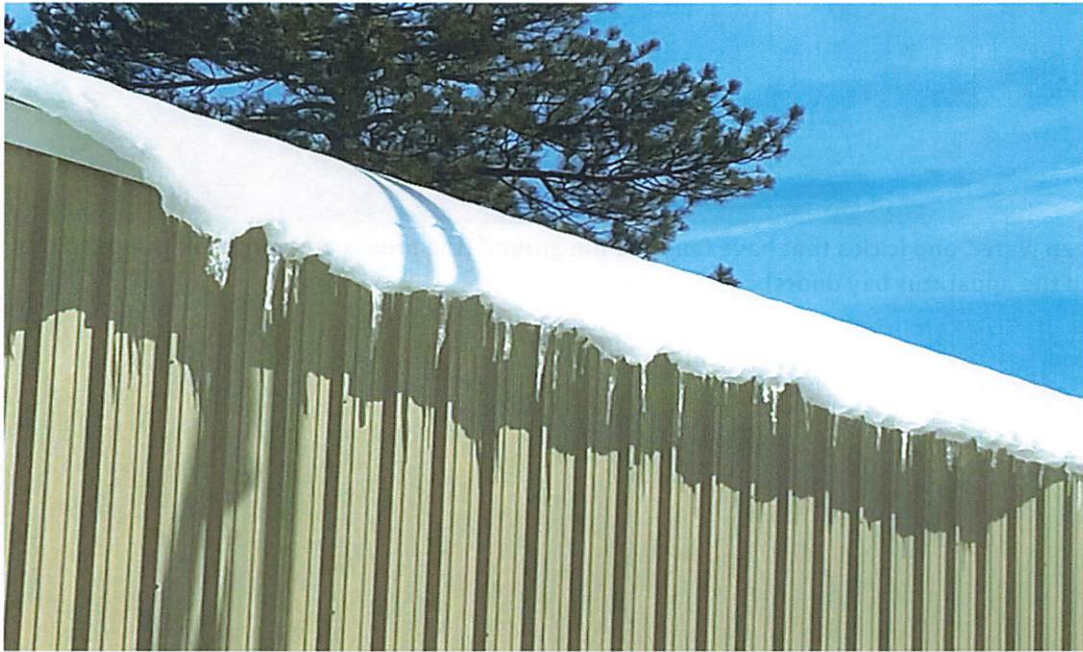
Snow and icicles hanging from roof's edge.
