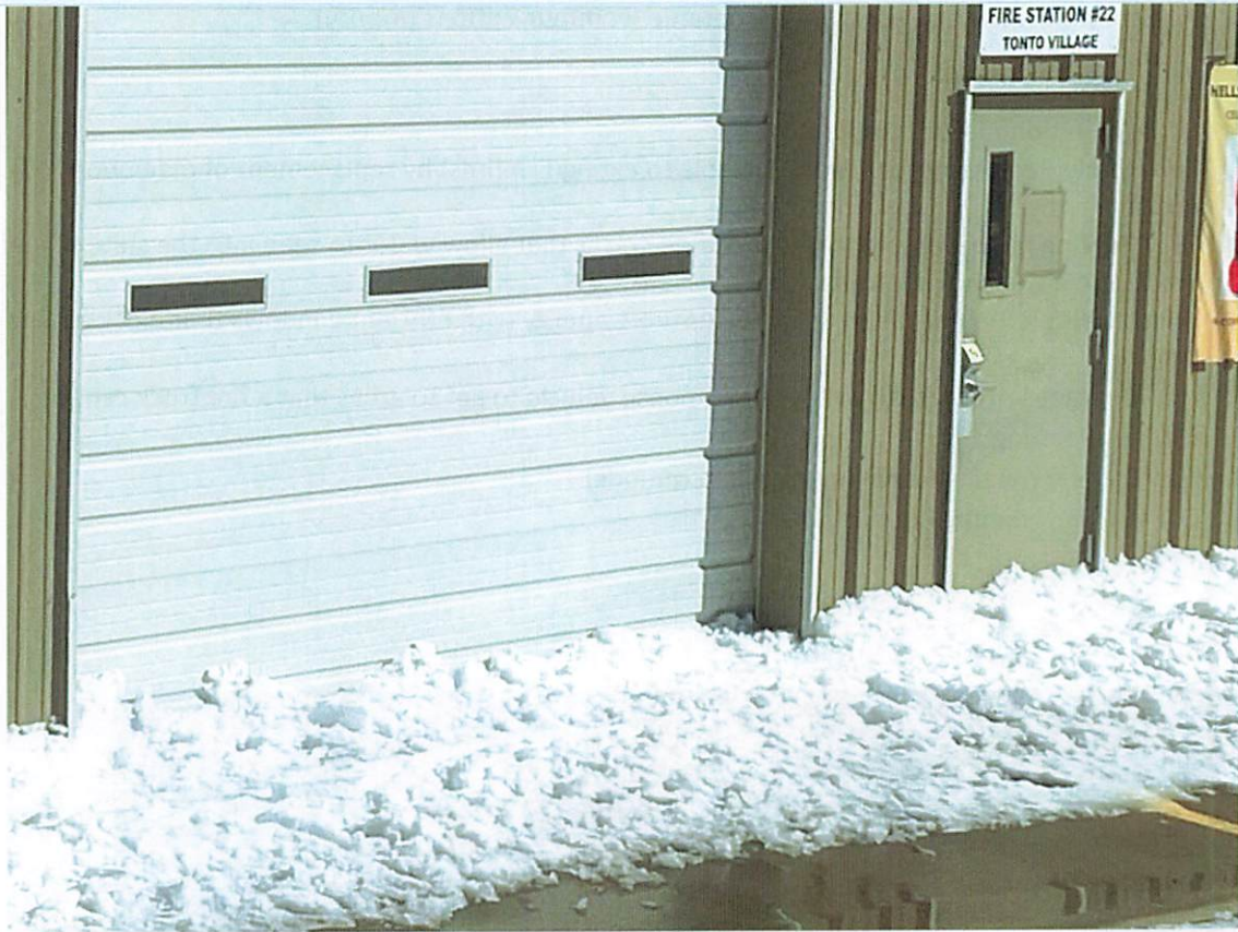
Snow, frozen water, and icicles that have fallen to the ground (the area is around the entrance to the station and the apparatus bay doors).
